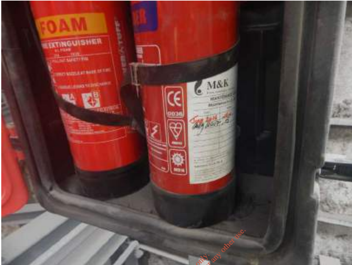
Figure 1.13: MRF Building: Fire Extinguisher (Inspection Date)
