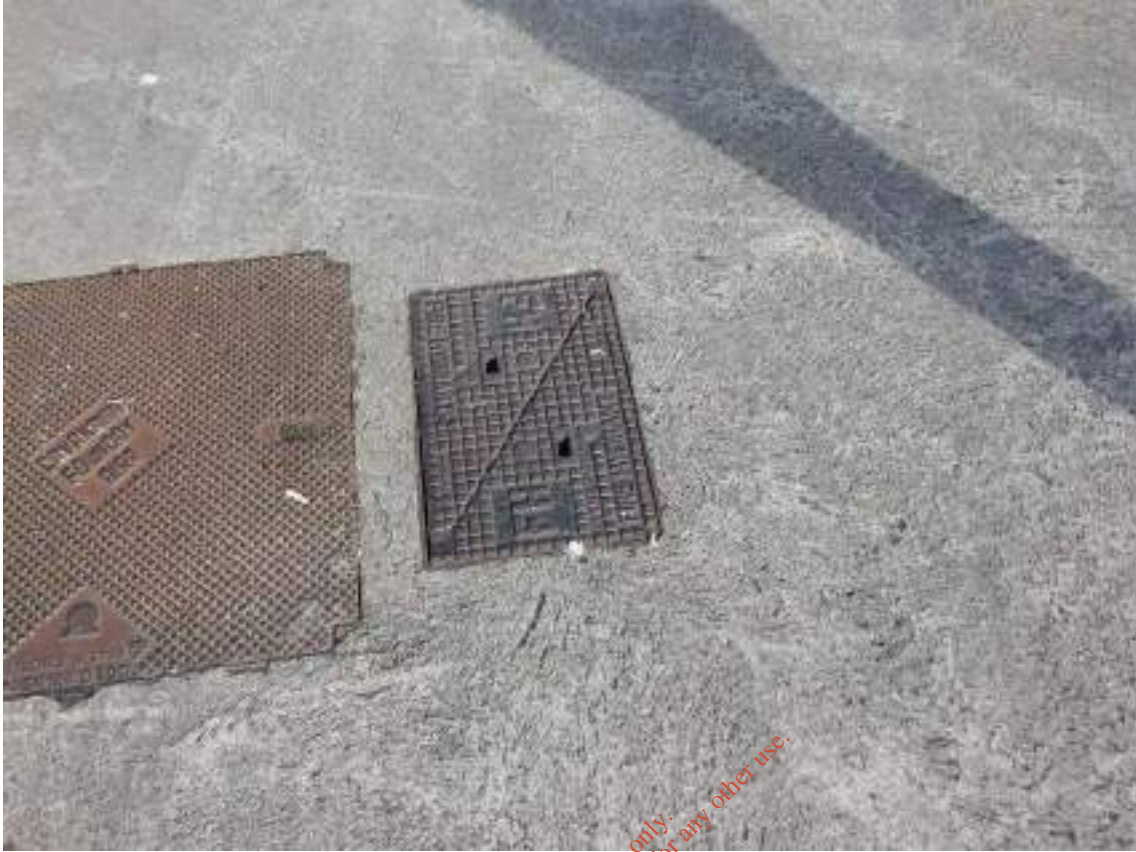
Figure 1.31: Yard Area: Hydrant 1 by Exit
