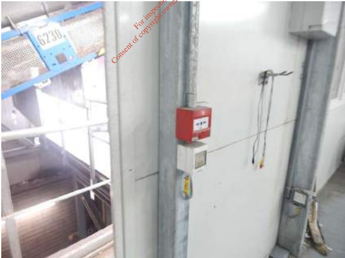
Figure 1.18: MRF Building: Break-glass Fire Alarm Unit
