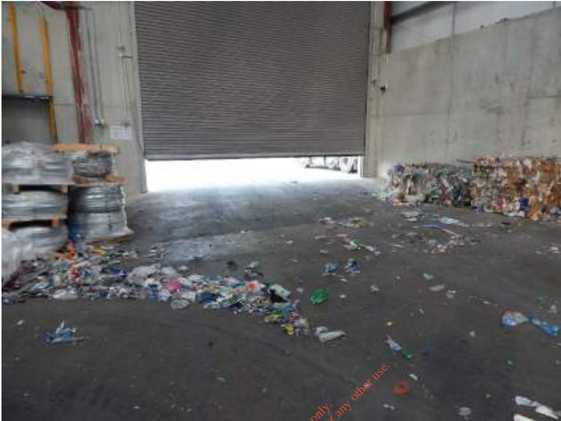
Figure 1.25: MRF Building: Fire Water Retention Ramp into and Out of MRF Building
