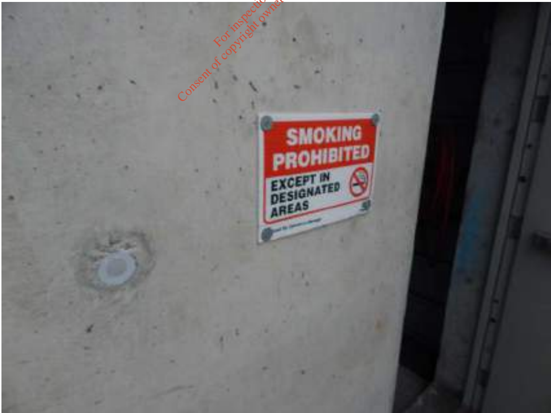
Figure 1.26: Yard Area: No Smoking Sign
