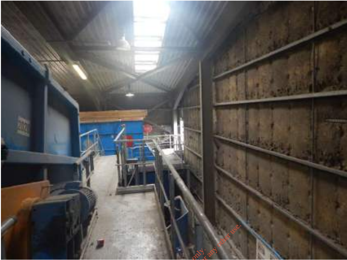
Figure 1.15: MRF Building: Fire Reel by Emergency Exit
