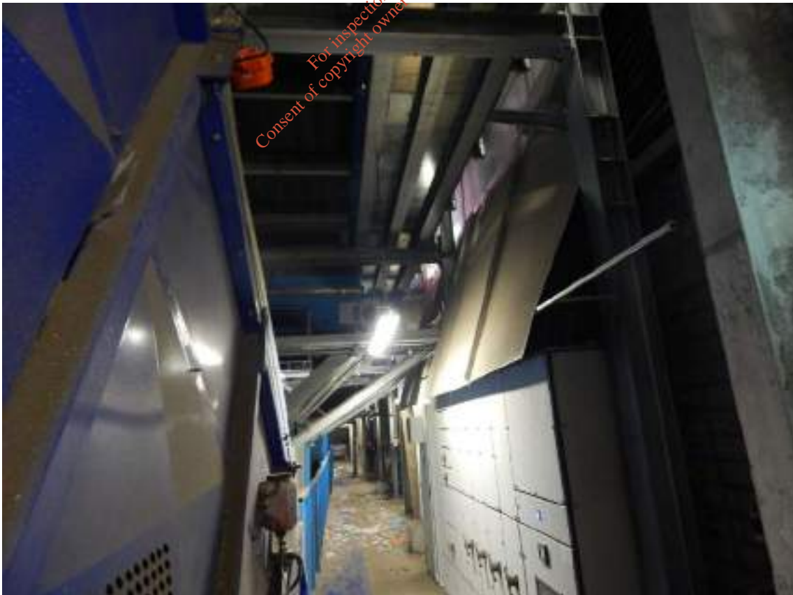
Figure 1.20: MRF Building: Flame Detection System by Electricity Controls
