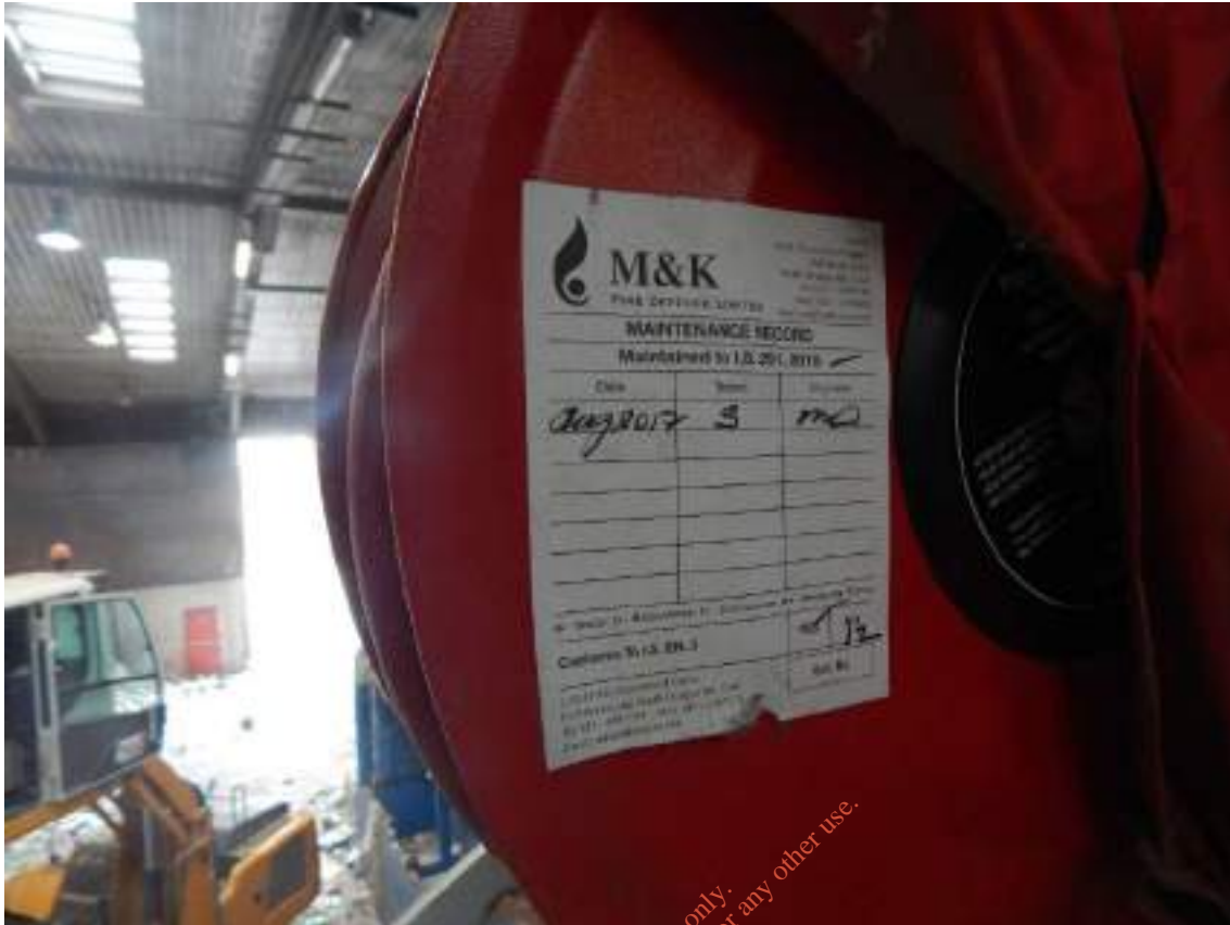
Figure 1.11: MRF Building: Fire Hose Reel (Inspection Date)
