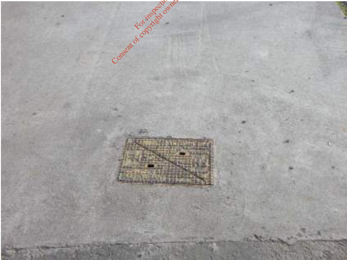
Figure 1.32: Yard Area: Hydrant 2 by Entrance
