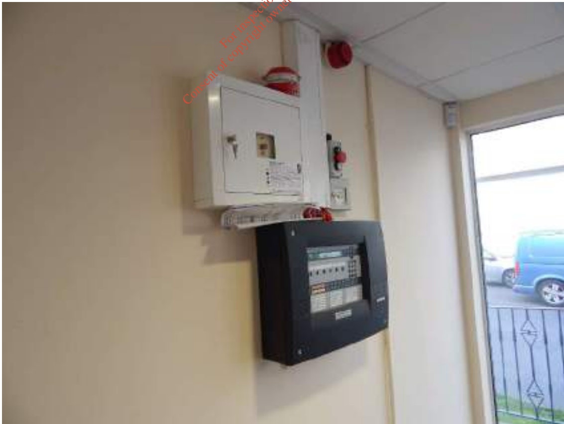
Figure 1.42: Administration Building: Fire Alarm Controls
