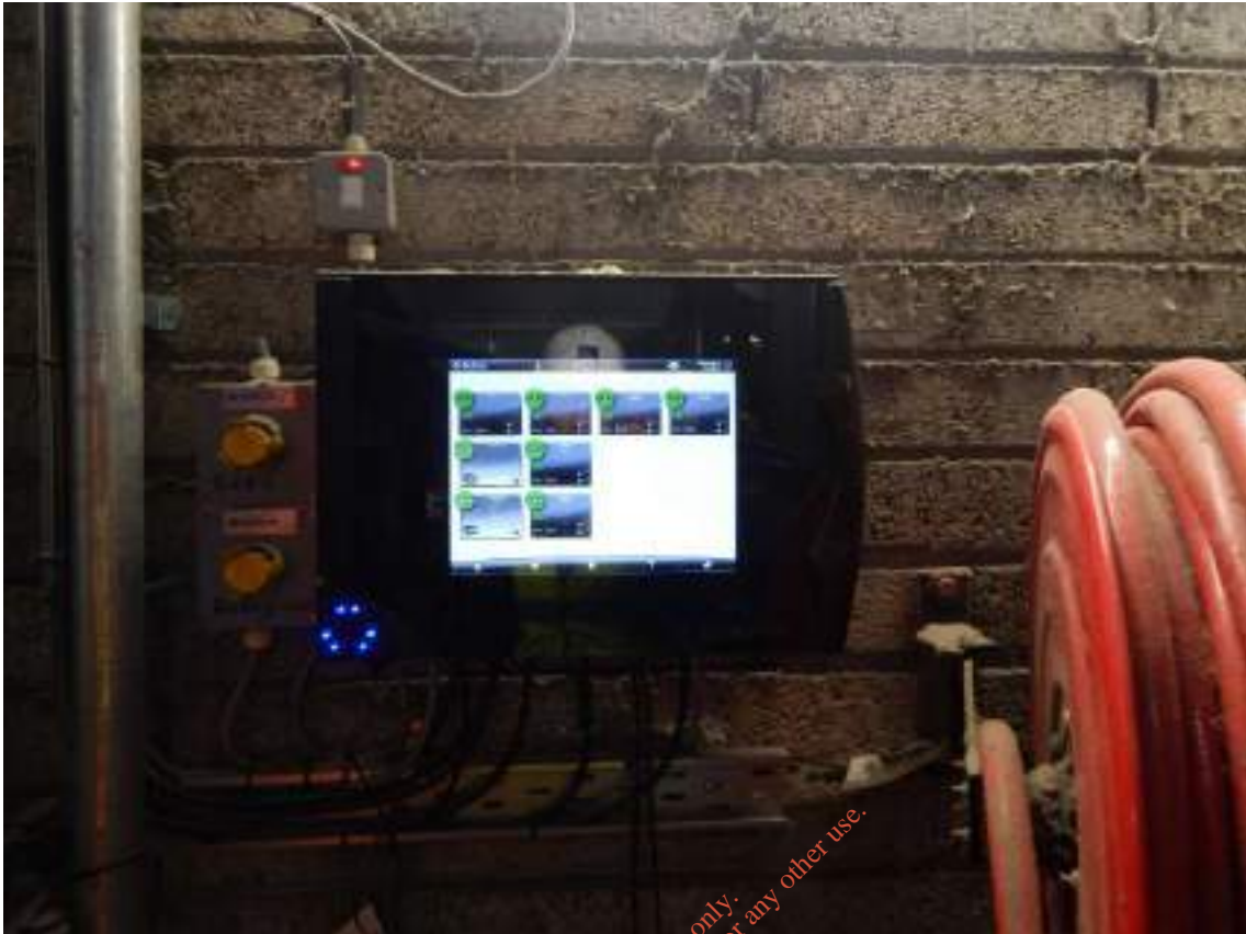
Figure 1.19: MRF Building: Flame Detection System Control Unit
