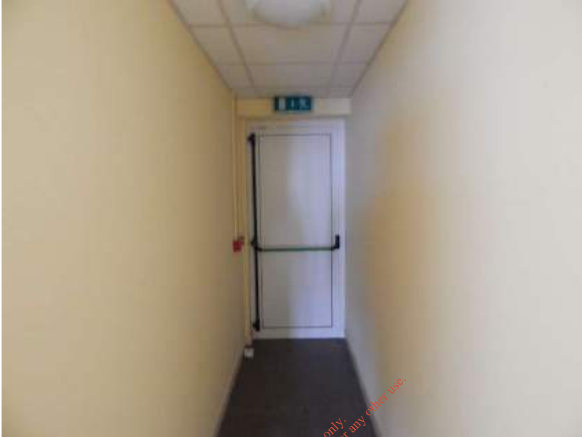
Figure 1.43: Administration Building: Push to Exit Door
