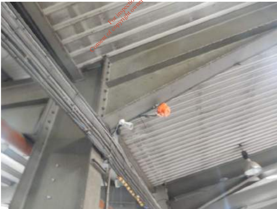
Figure 1.12: MRF Building: Flame Detection System
