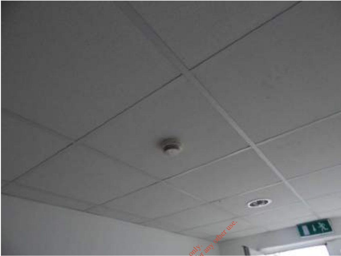
Figure 1.39: Administration Building: Smoke Detector & Emergency Exit
