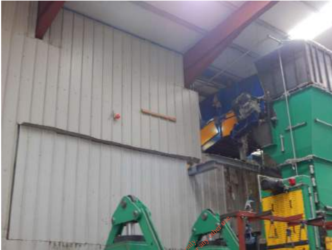
Figure 1.23: MRF Building: Flame Detection System & inbuilt Sprinkler System
