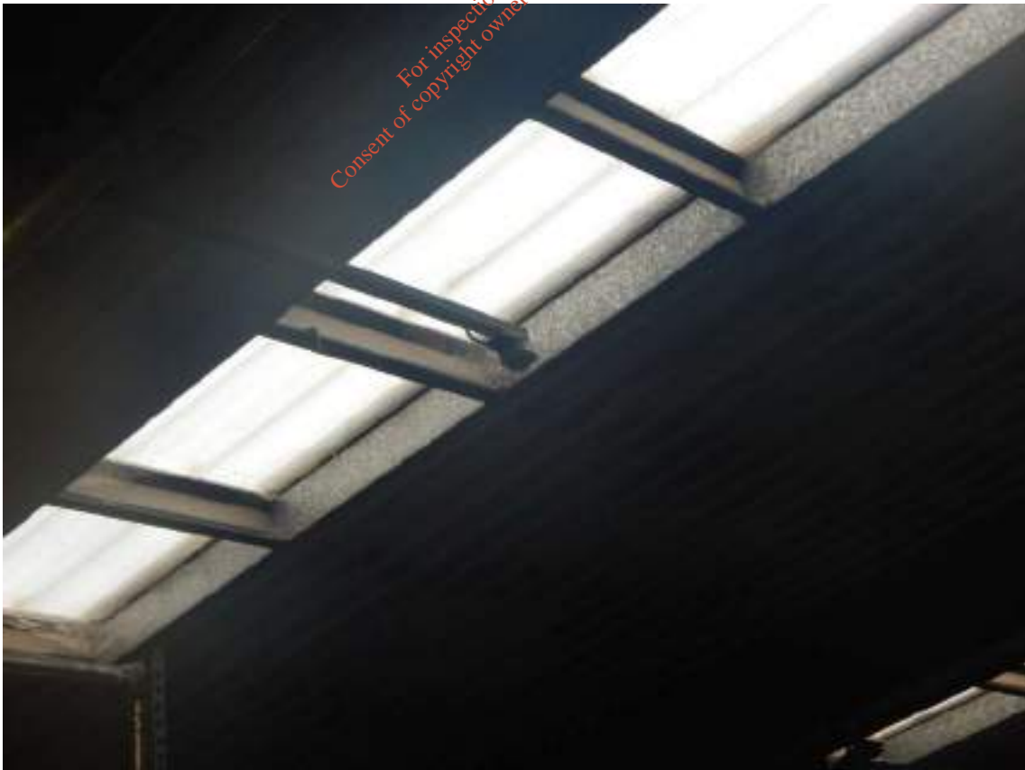
Figure 1.16: MRF Building: Smoke Detector
