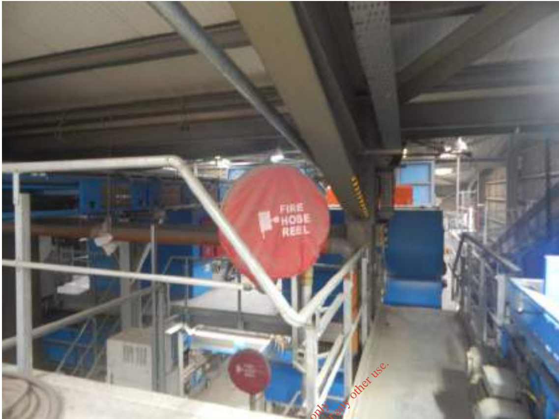
Figure 1.17: MRF Building: Fire Hose Reels by Machinery
