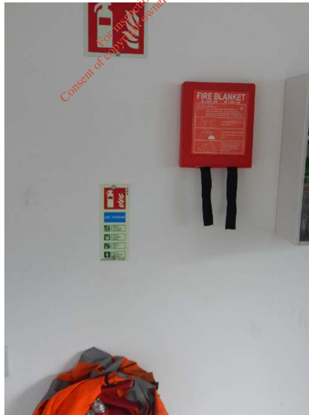
Figure 1.38: Administration Building: Canteen Fire Blanket & Extinguisher
