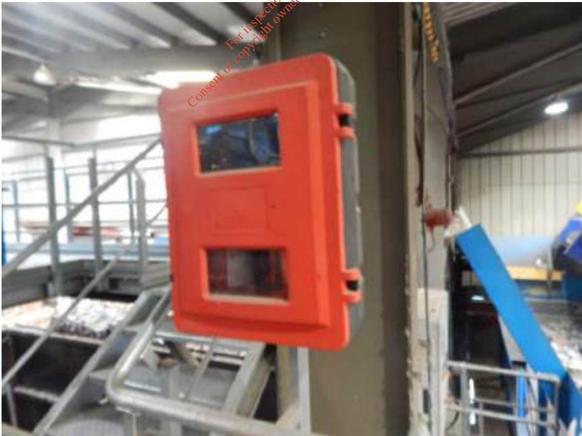
Figure 1.10: MRD Building: Fire Extinguisher storage
