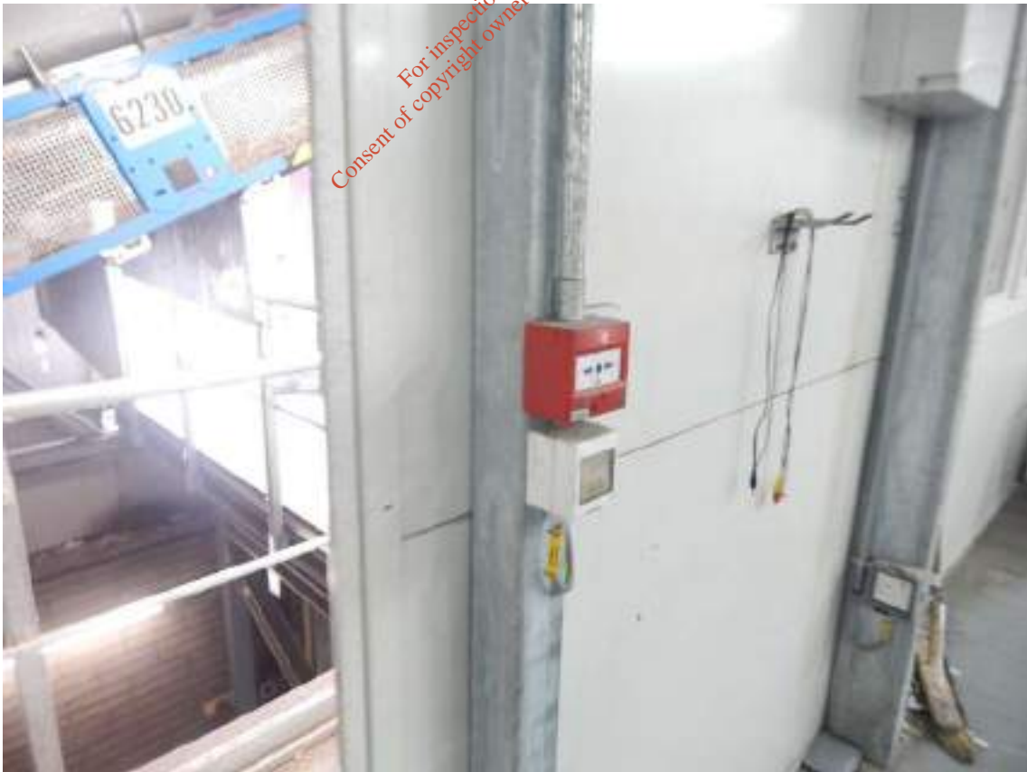
Figure 1.18: MRF Building: Break-glass Fire Alarm Unit
