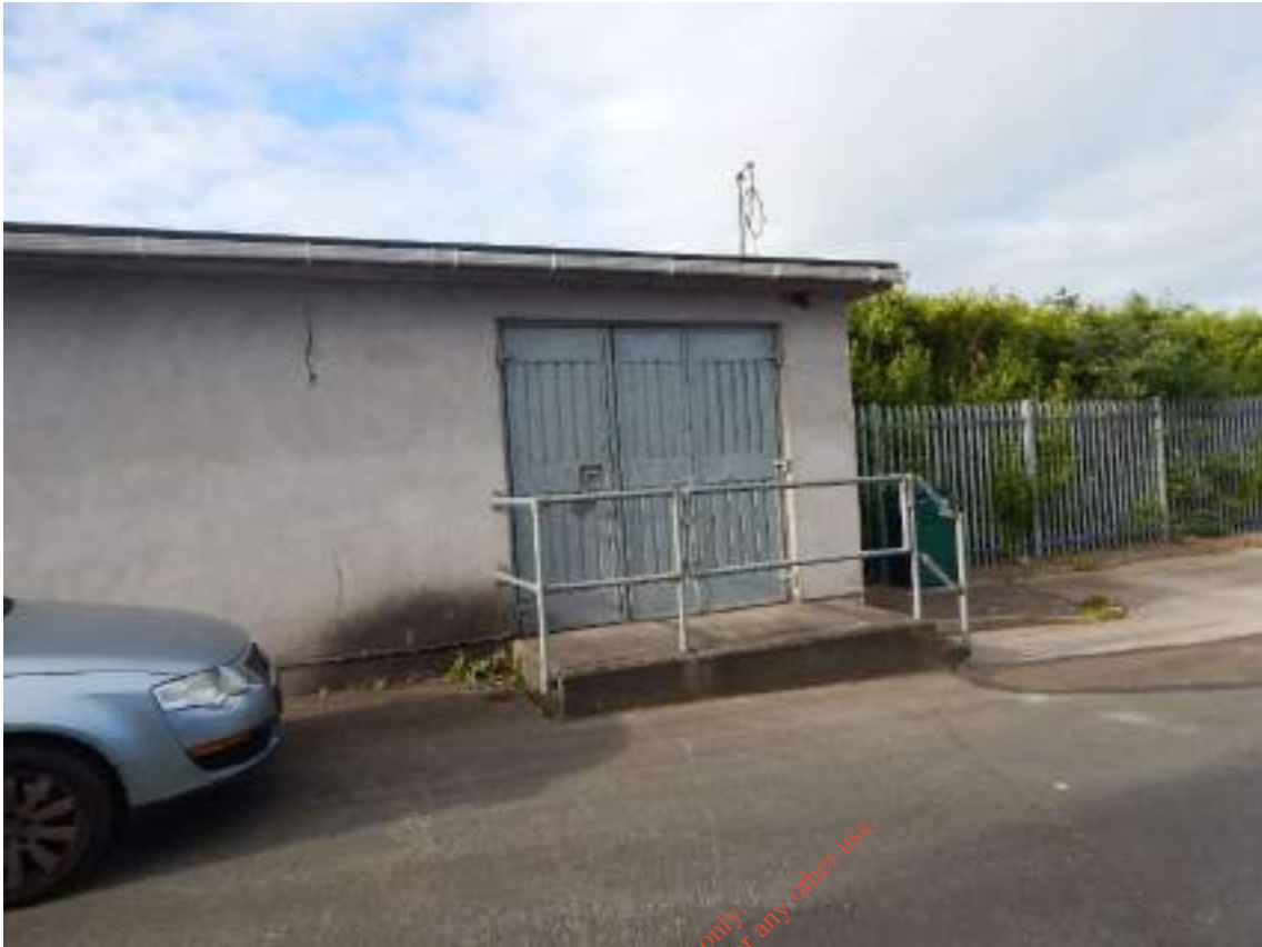
Figure 1.27: Yard Area: ESB Substation
