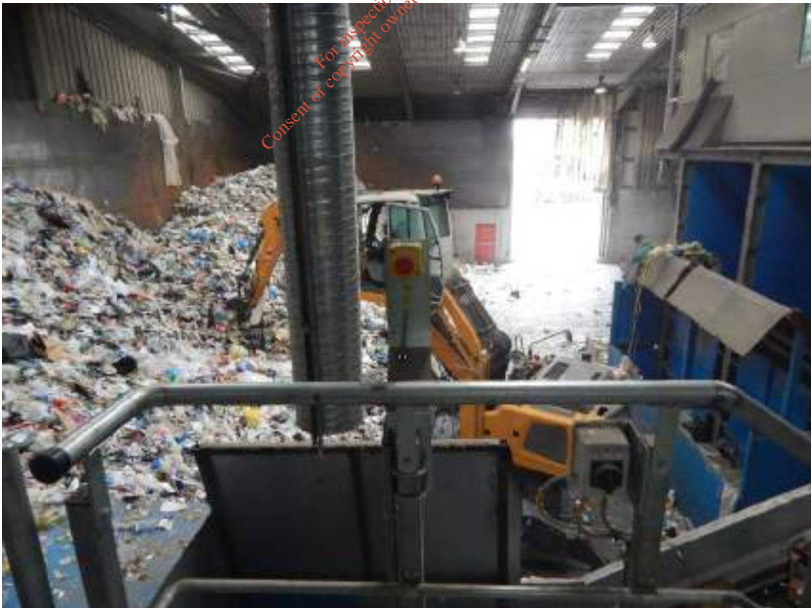
Figure 1.14: MRF Building: Emergency Stop Button
