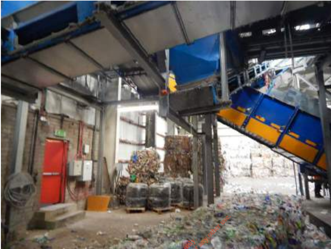
Figure 1.21: MRF Building: Flame Detection System by Baler
