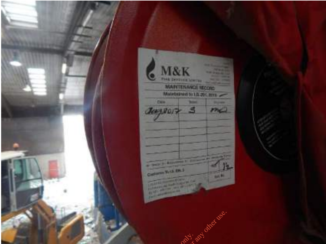
Figure 1.11: MRF Building: Fire Hose Reel (Inspection Date)
