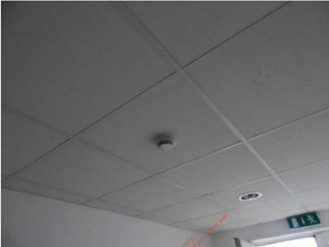
Figure 1.39: Administration Building: Smoke Detector & Emergency Exit
