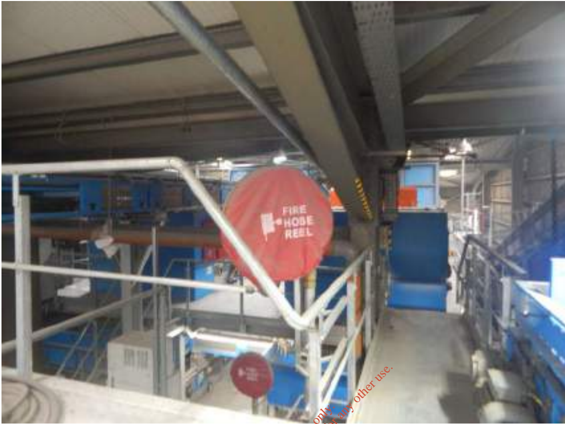
Figure 1.17: MRF Building: Fire Hose Reels by Machinery
