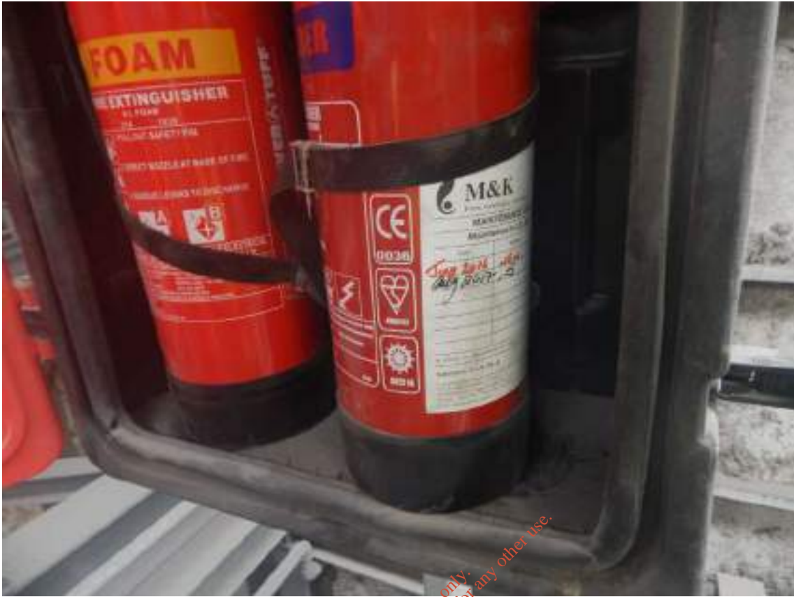
Figure 1.13: MRF Building: Fire Extinguisher (Inspection Date)
