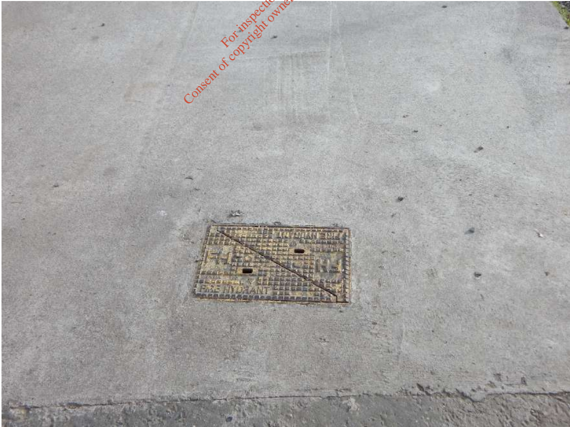
Figure 1.32: Yard Area: Hydrant 2 by Entrance
