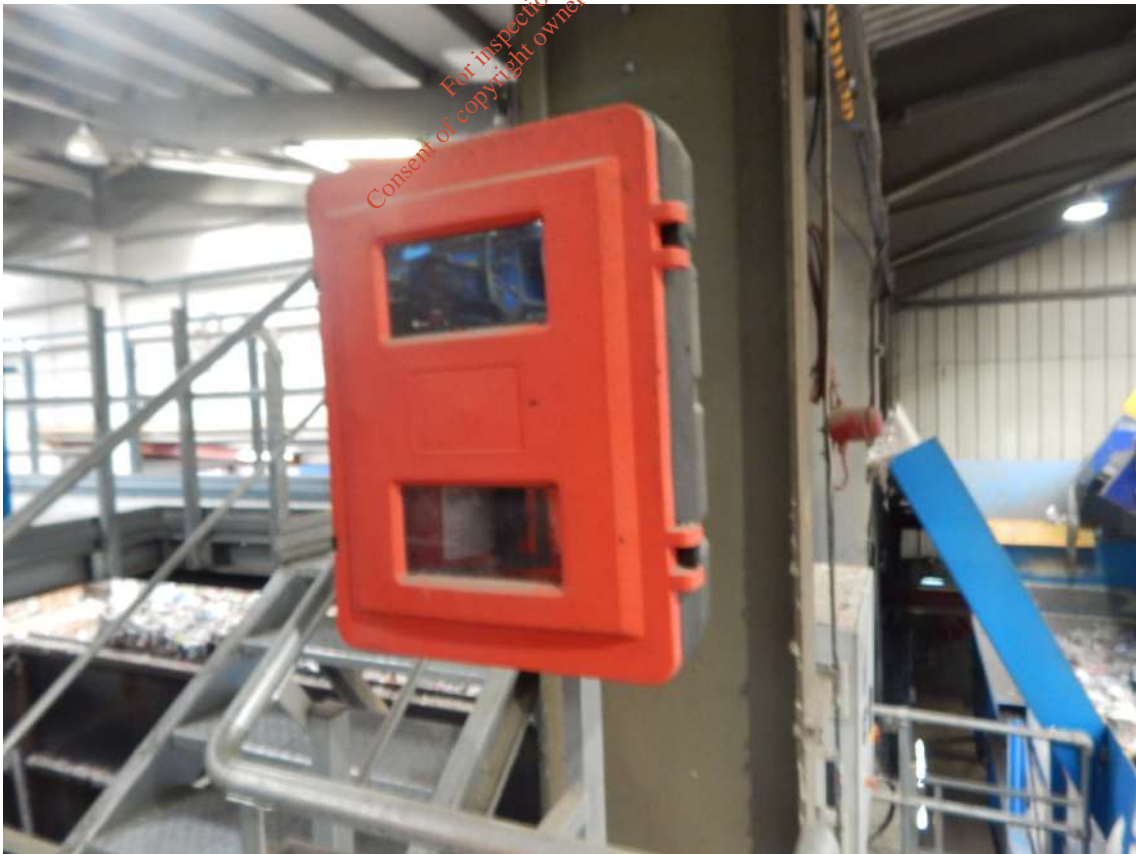
Figure 1.10: MRD Building: Fire Extinguisher storage
