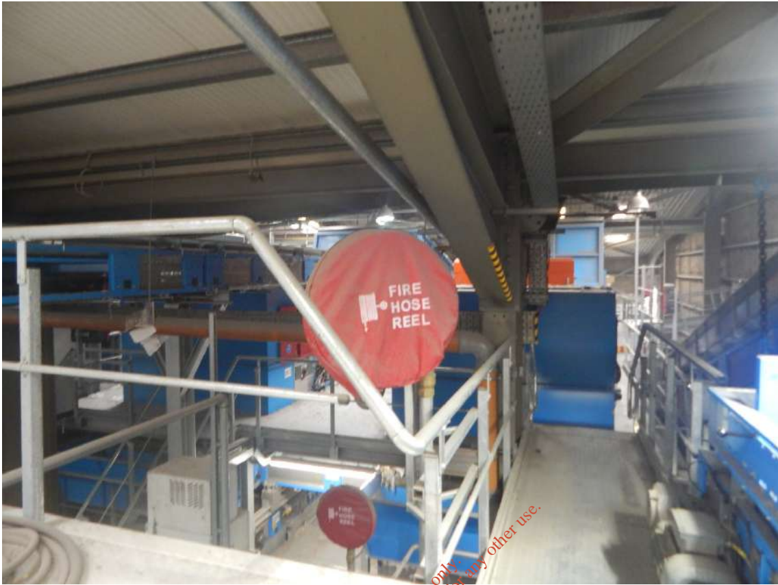
Figure 1.17: MRF Building: Fire Hose Reels by Machinery
