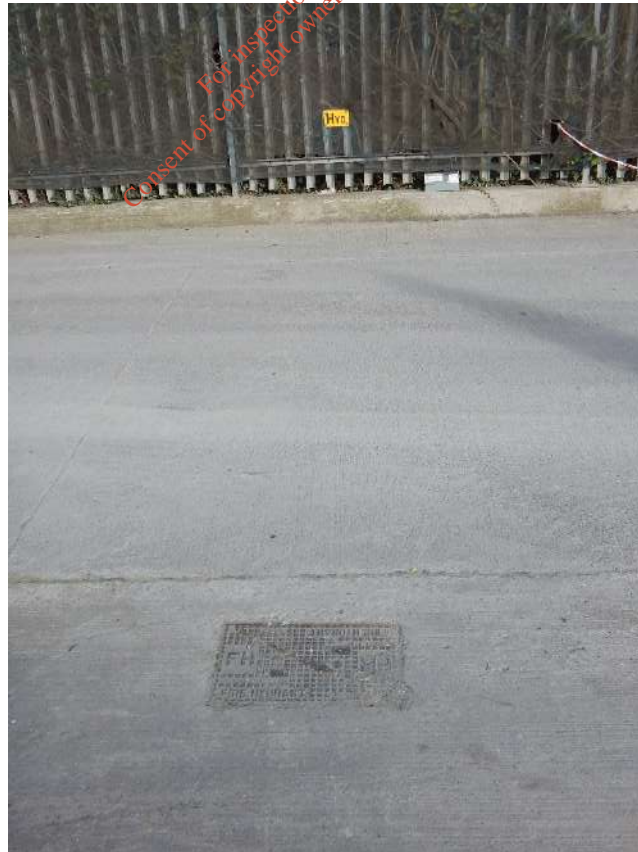
Figure 1.34: Yard Area: Hydrant 4 by North East Corner of MRF Building
