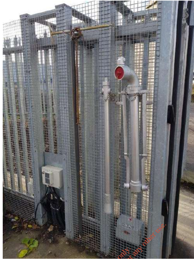
Figure 1.41: Yard Area: Fire Hydrant Fittings
