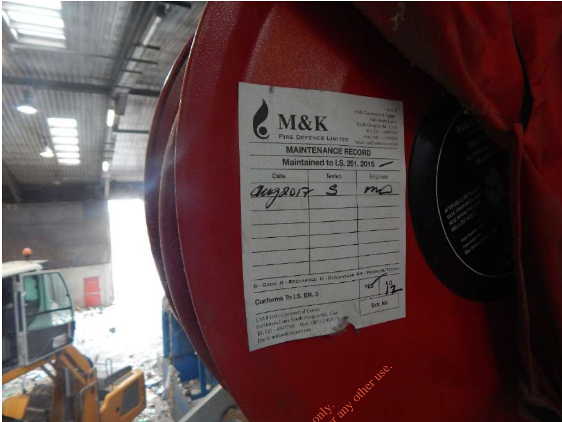
Figure 1.11: MRF Building: Fire Hose Reel (Inspection Date)
