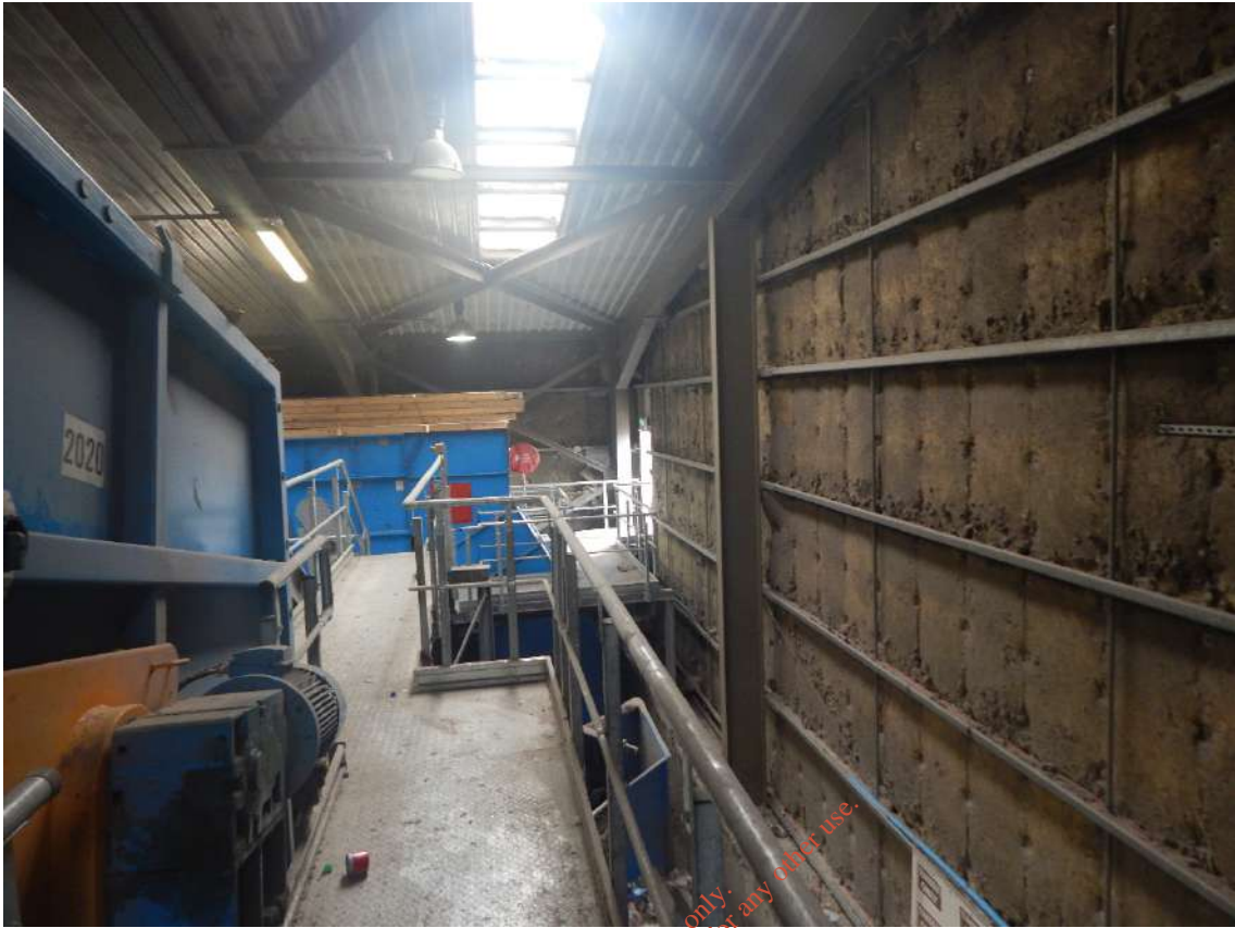
Figure 1.15: MRF Building: Fire Reel by Emergency Exit
