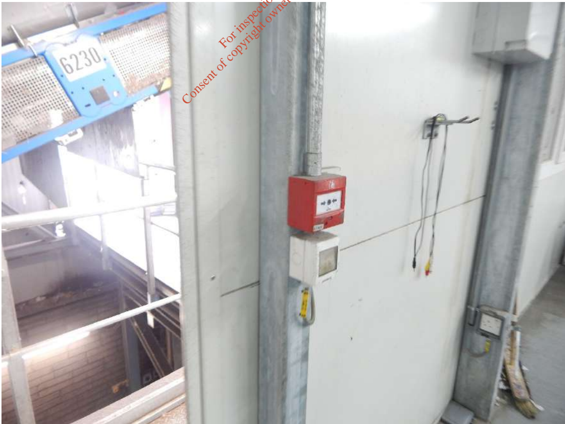
Figure 1.18: MRF Building: Break-glass Fire Alarm Unit
