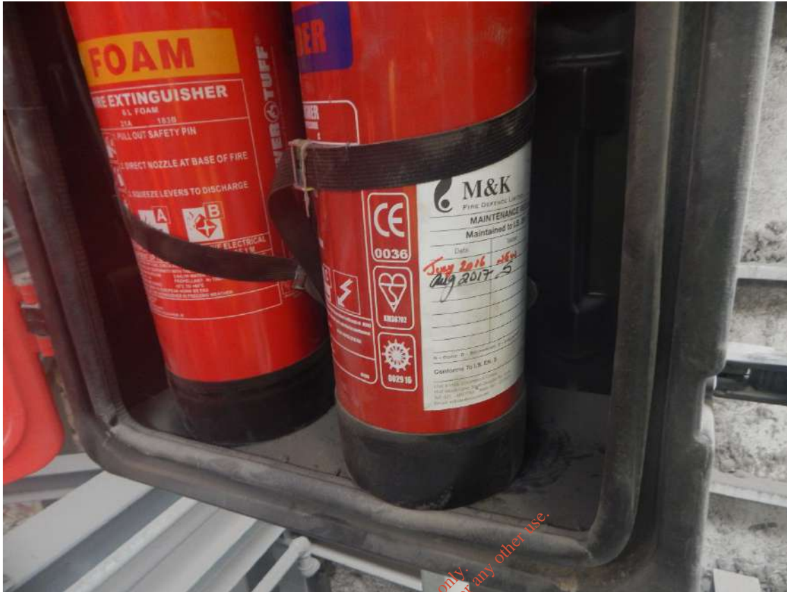
Figure 1.13: MRF Building: Fire Extinguisher (Inspection Date)
