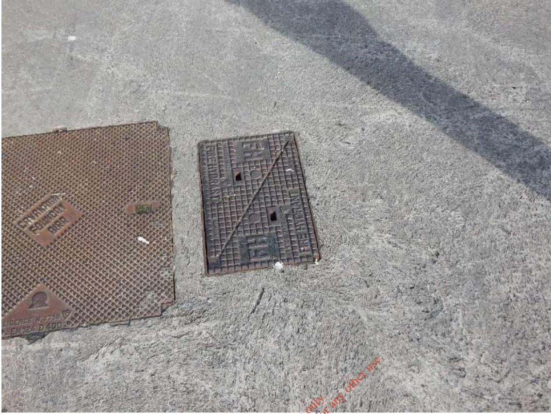
Figure 1.31: Yard Area: Hydrant 1 by Exit
