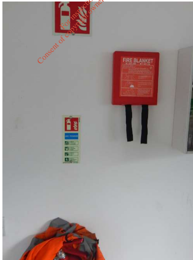
Figure 1.38: Administration Building: Canteen Fire Blanket & Extinguisher
