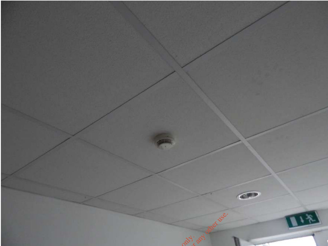
Figure 1.39: Administration Building: Smoke Detector & Emergency Exit
