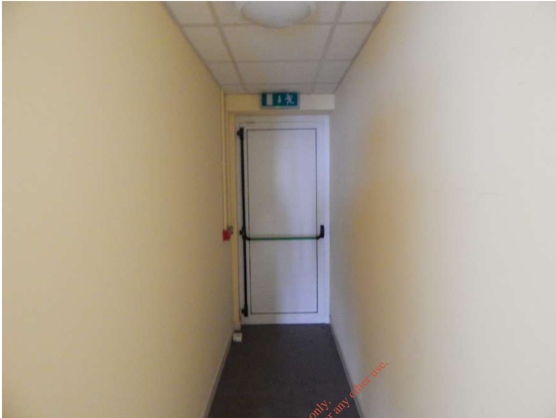
Figure 1.43: Administration Building: Push to Exit Door
