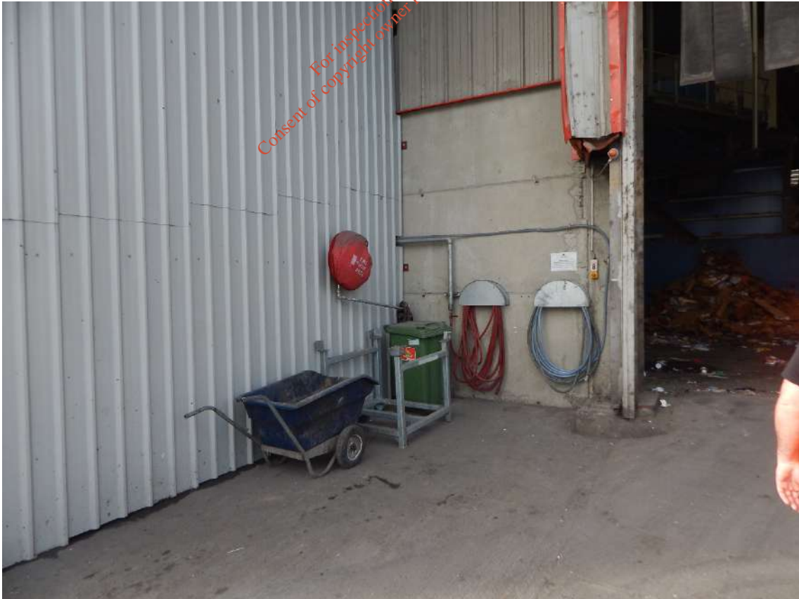
Figure 1.8: Yard Area: Fire Fighting Equipment by Incoming MDR Roller Door
