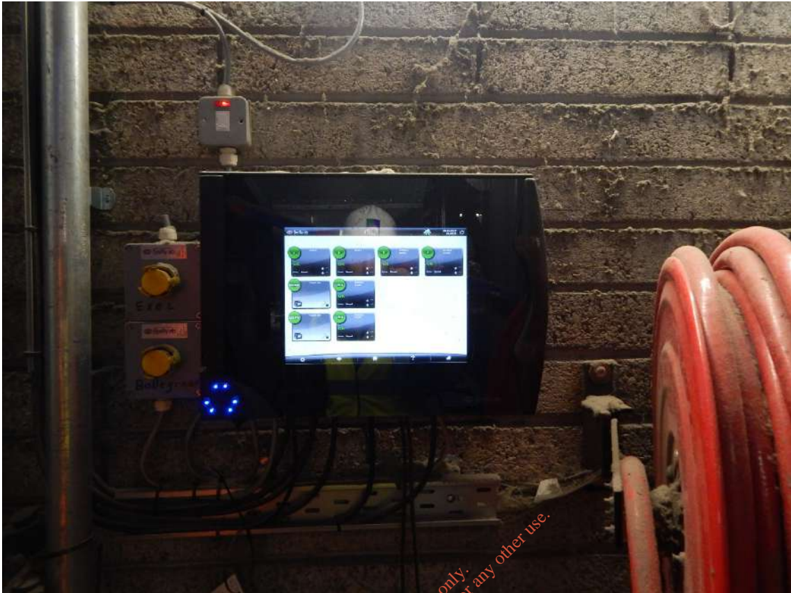
Figure 1.19: MRF Building: Flame Detection System Control Unit
