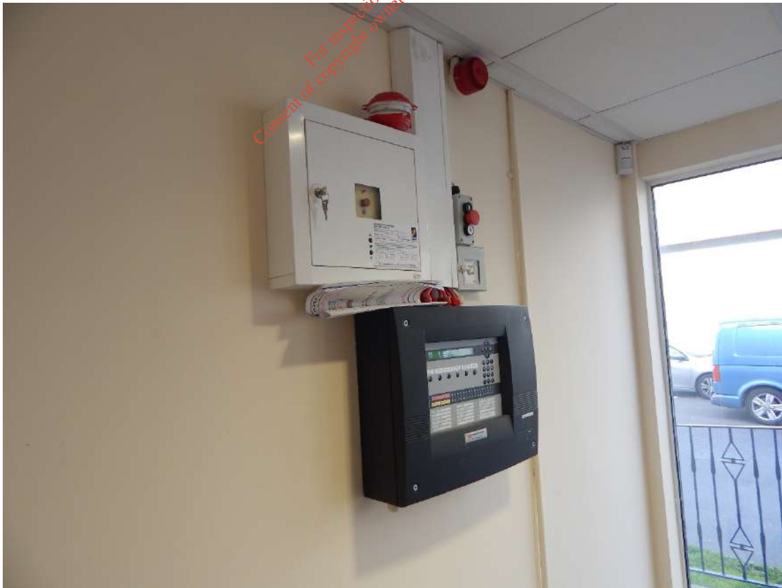
Figure 1.42: Administration Building: Fire Alarm Controls
