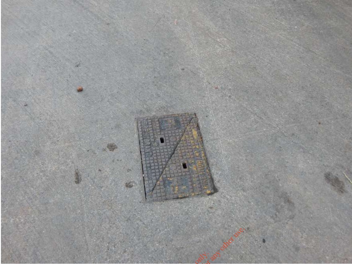
Figure 1.33: Yard Area: Hydrant 3 by South East Corner of Site
