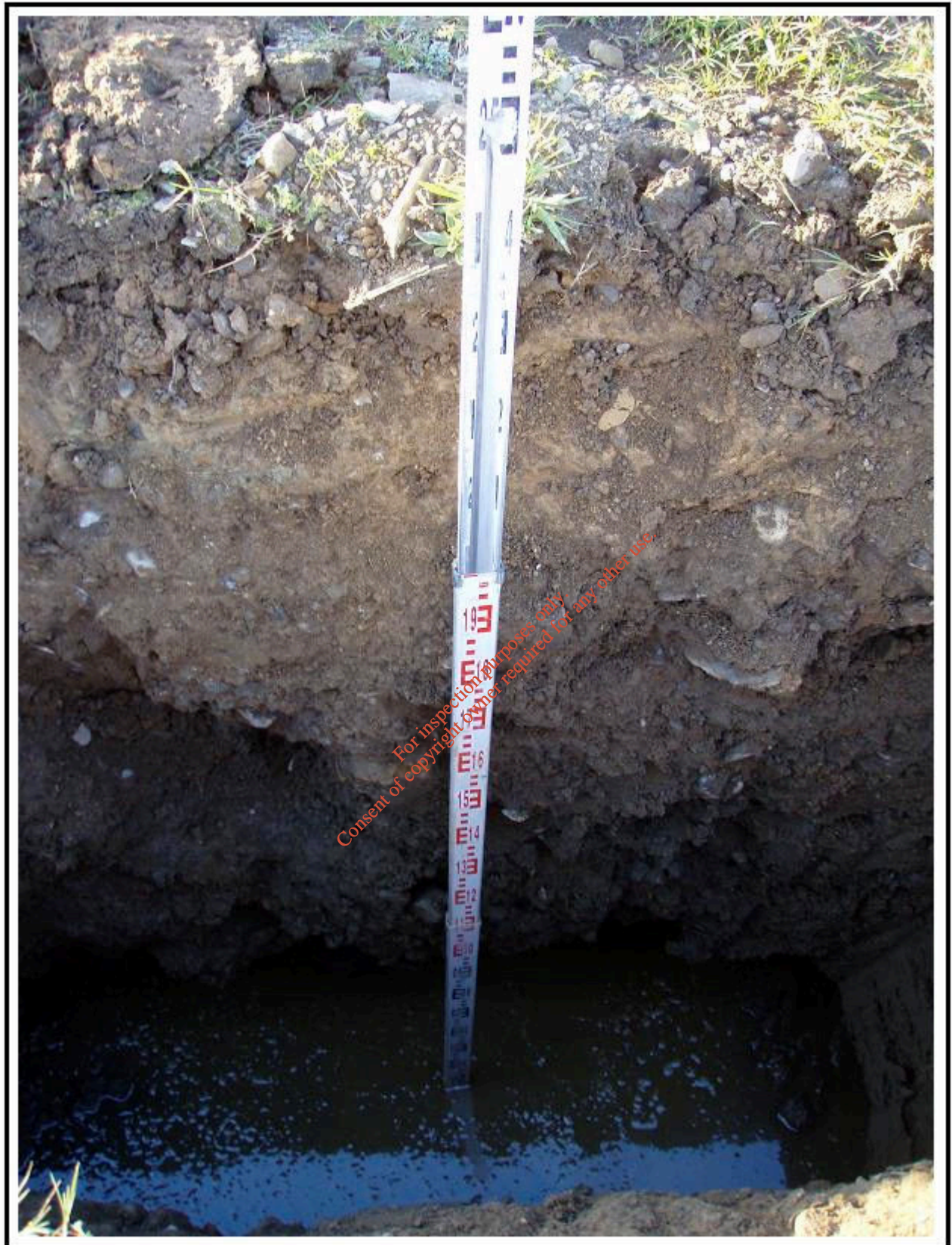
Plate A7: Profile of shallow topsoil overlying subsoil in trial hole no. 7. The water table seeps into this hole and rests at 2.04m depth below surface. See the complete absence of waste material and the preponderance of 'clean' imported subsoil here.
