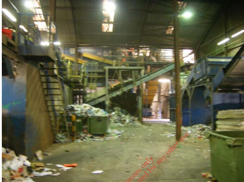
Figure 2.3: Dry recyclable mechanical processing area
