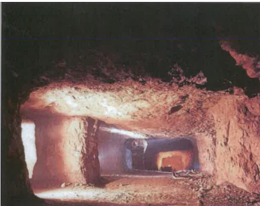
Figure 2.9: Typical rooms and pillars, Galmoy Mine prior to backfilling. The competent rock conditions shown are an example of good rockmass conditions expected in the K2, K and R zones.
