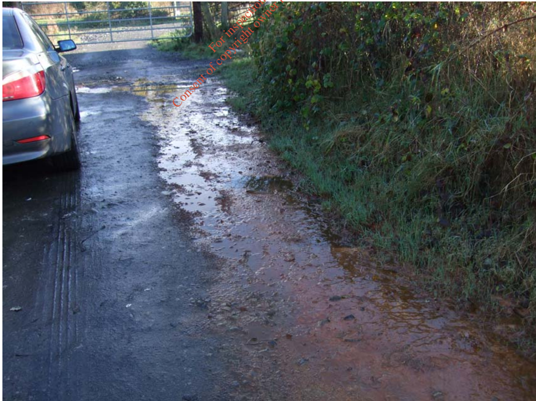
Photo 10: Leachate runoff flowing across the cul-de-sac to stream.
