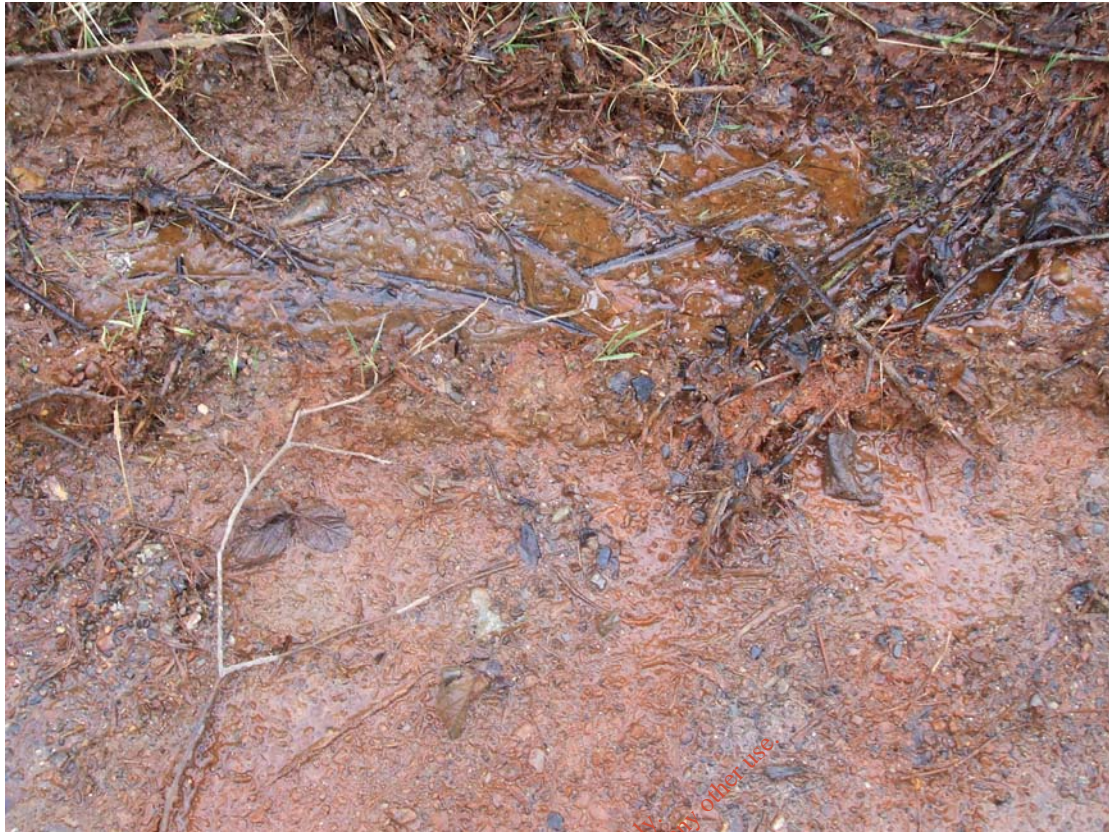
Photo 11: "Reddish" leachate on road pavement.
