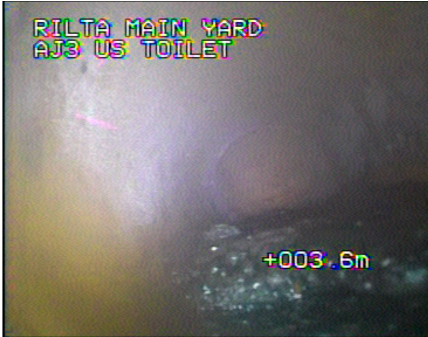
Photo: 10_5A, MPEG #: 280217_1, 00:00:35 3.6m, Settled deposits, fine, 15% cross-sectional area loss
