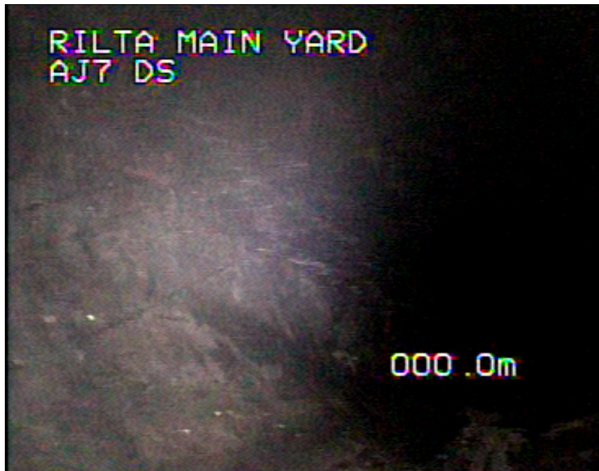
Photo: 45_9A, MPEG #: 280217_1, 00:00:00 39.59m, Other obstacles built into structure, from 1 to 3 o'clock, 75% cross-sectional area loss
