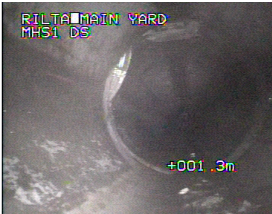
Photo: 27_4A, MPEG #: 280217_1, 00:00:47 1.5m, Sealing ring intruding, from 9 to 12 o'clock
