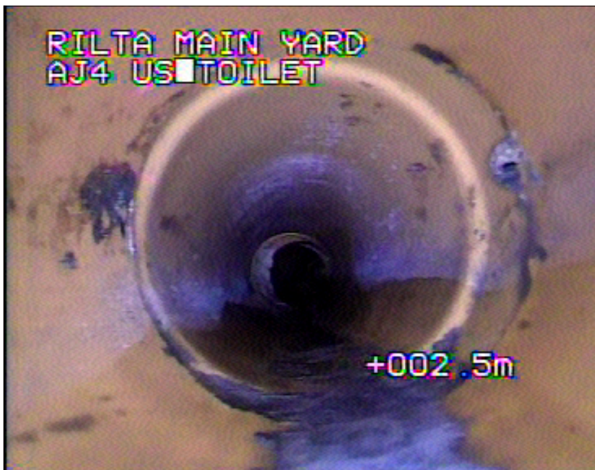
Photo: 13_4A, MPEG #: 280217_1, 00:00:36 2.5m, Open joint, medium
