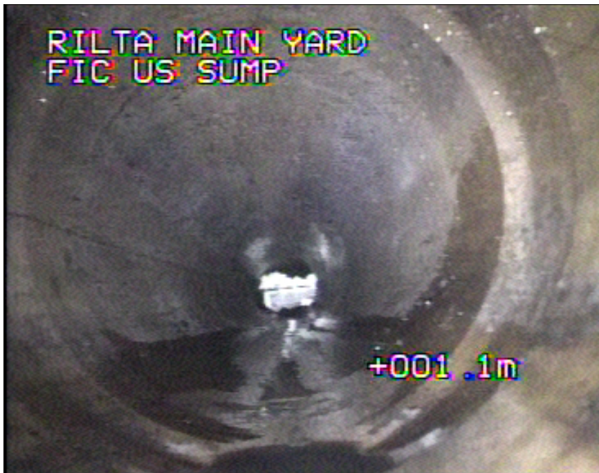
Photo: 19_3A, MPEG #: 280217_1, 00:00:27 1.1m, Open joint, medium
