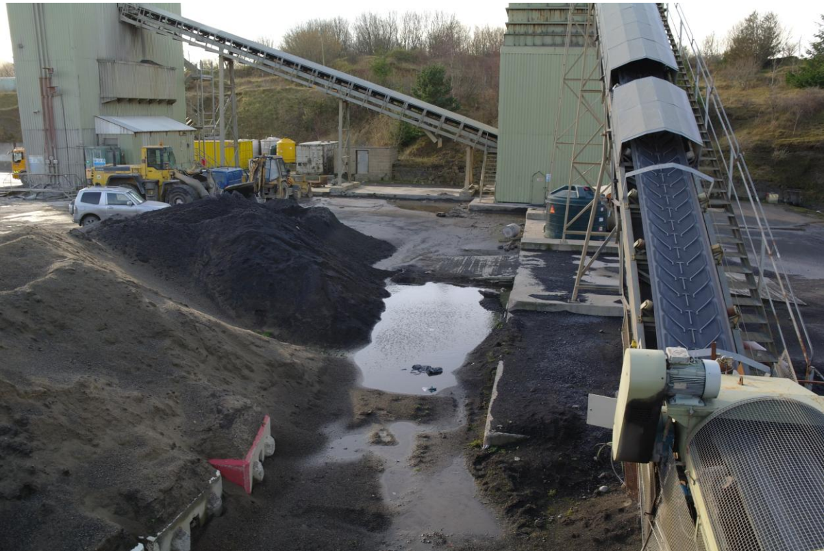
Photo 5 – Yard Drainage Impeded by Concrete Platform
