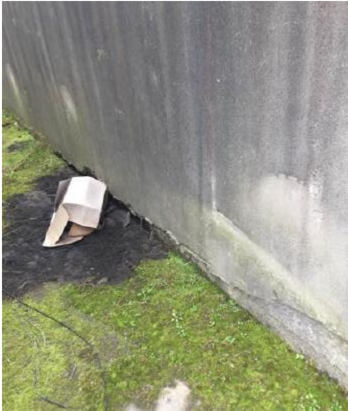
Figure 2-2 Leak from base of bund wall
