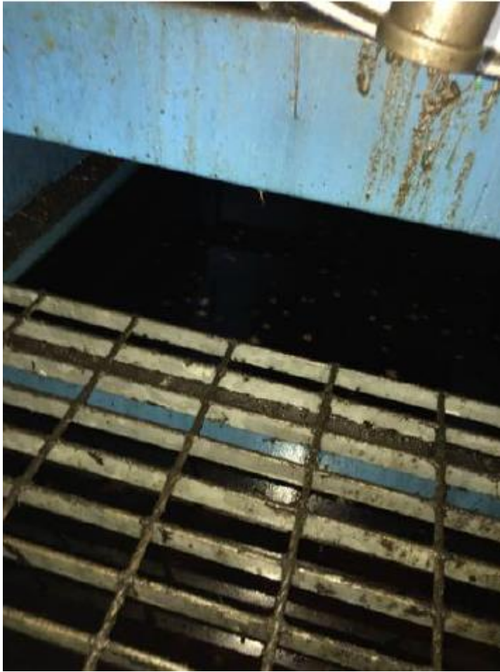
Figure 2-5 Sump of bund full of oil.
