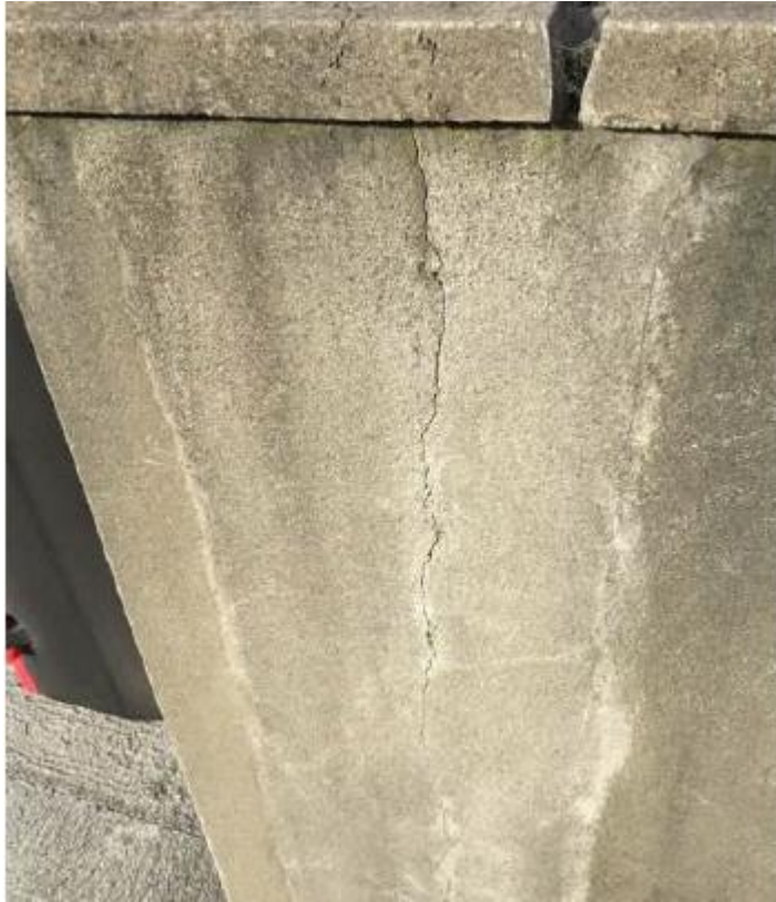
Figure 2-1 Example of crack in bund wall
