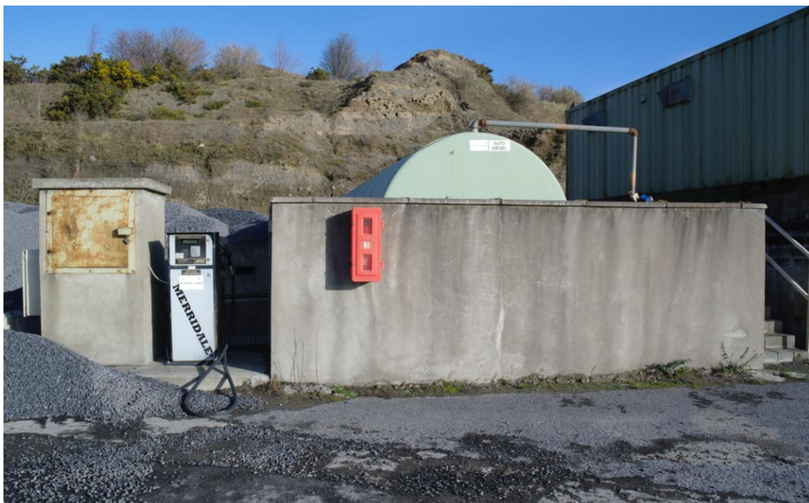
Photo 1 - Bunded 70,000 litre Diesel Tank
