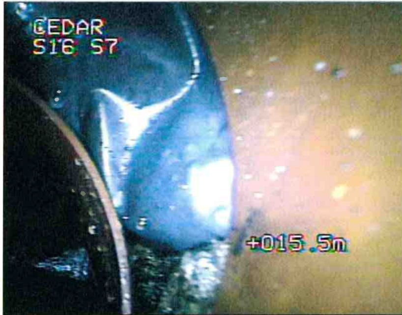
Photo: 49_6A, MPEG #: 051216_1, 00:02:41 15.4m, Joint displaced, large
