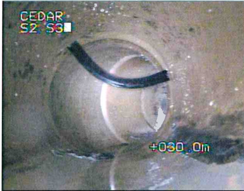
Photo: 23_3A, MPEG #: 051216_1, 00:04:31 30m, Sealing ring intruding, from 11 to 3 o'clock
