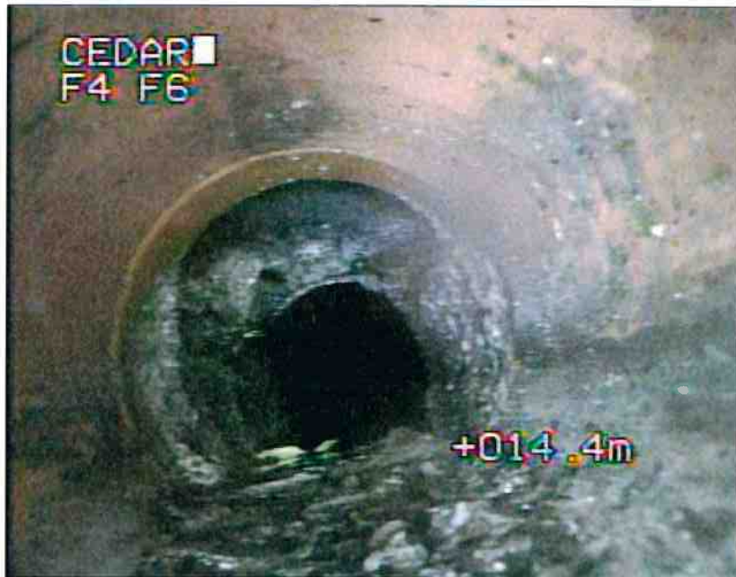
Photo: 7_6A, MPEG #: 051216_1, 00:02:24 14.3m, Settled deposits, hard or compacted, 10% cross-sectional area loss
