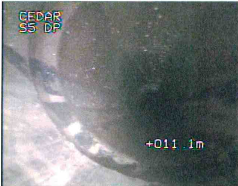
Photo: 27_9A, MPEG #: 051216_1, 00:01:44 11.1m, Open joint, medium
