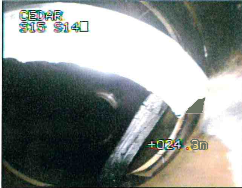
Photo: 47_6A, MPEG #: 051216_1, 00:02:39 24.3m, Sealing ring intruding, from 10 to 6 o'clock
