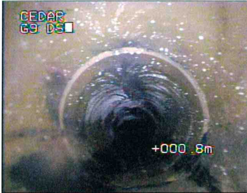
Photo: 22_3A, MPEG #: 051216_1, 00:00:12 0.9m, Sealing ring intruding, from 5 to 7 o'clock
