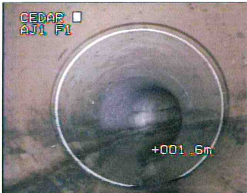
Photo: 1_6A, MPEG #: 051216_1, 00:00:00 7.71m, Finish node type, manhole reference number: F1
