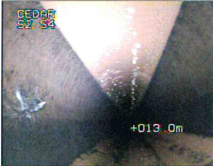
Photo: 24_10A, MPEG #: 051216_1, 00:02:35 13m, Surface damage, other, from 8 to 9 o'clock
