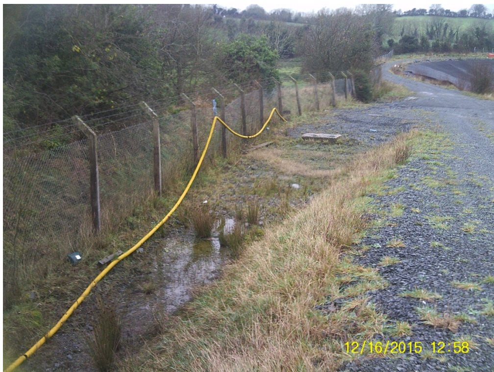
Figure 15 – Ponding in Drain at Toe of Northwest Slope of Cell 3 (facing northwest)
