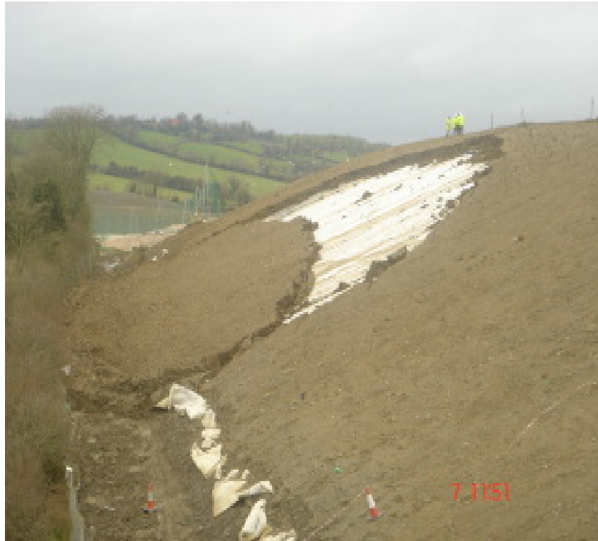
Figure 7 – Northwest Slope of Cell 1 in 2006 following shallow slope failure (facing northwest)
