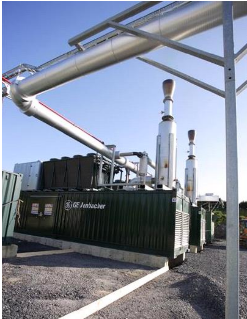
Figure 3-2: Landfill Gas Utilisation Plant at Arthurstown
