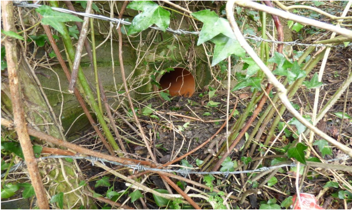
Figure 1: Overflow Discharge Pipe from Moulden Bridge Pumping Station Rathoath
