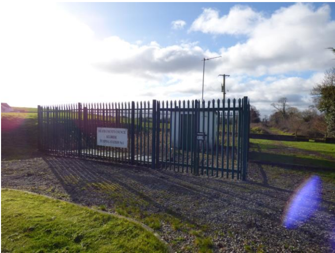
Figure 2 Cherry Tree Drive Pumping Station
