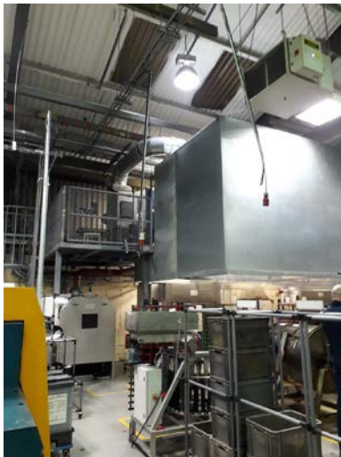
Fig.3 Enclosure and abatement unit for one of the installation's four vents for tempering ovens.
