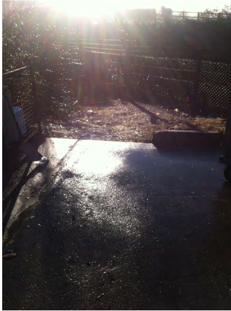
Photograph 9: Soil Sample Location at Missing Curbing at South Boundary
