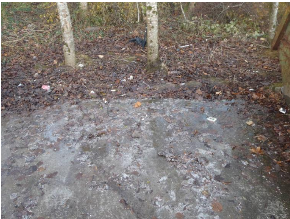
Photo 4: close-up of eastern edge of concrete pad (lower yard) where kerbing was absent and a white-coloured slime deposit was evident on the concrete surface.
