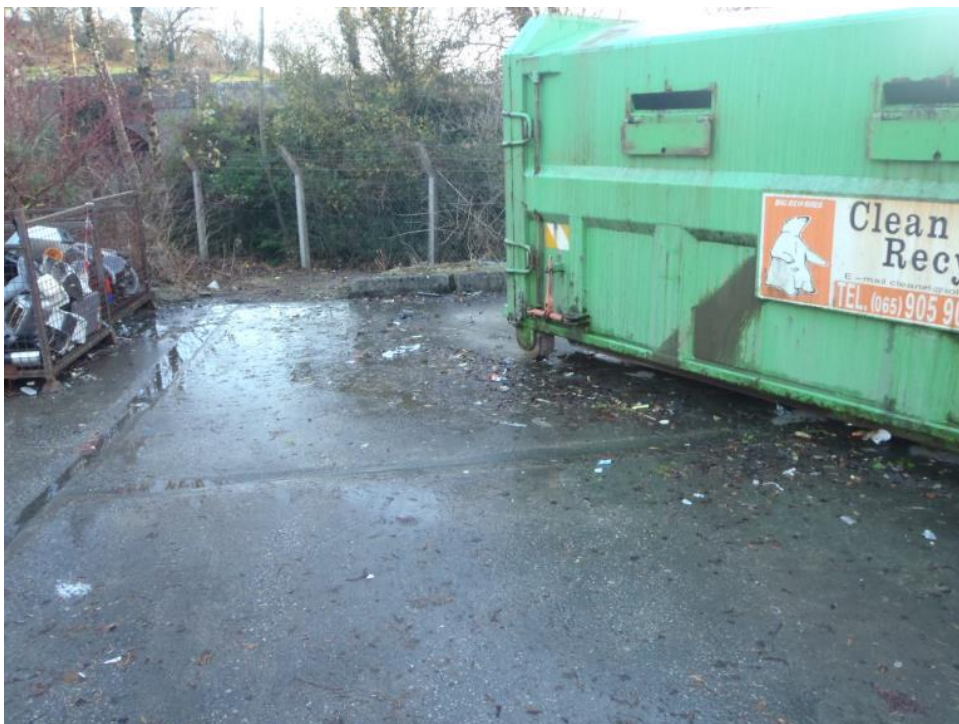
Photo 6: general view of the southern edge of the lower yard (facing south). Note the absence of kerbing at the edge of the concrete pad beside the WEEE receptacles, and the seepage of run-off moving towards the unpaved area.
