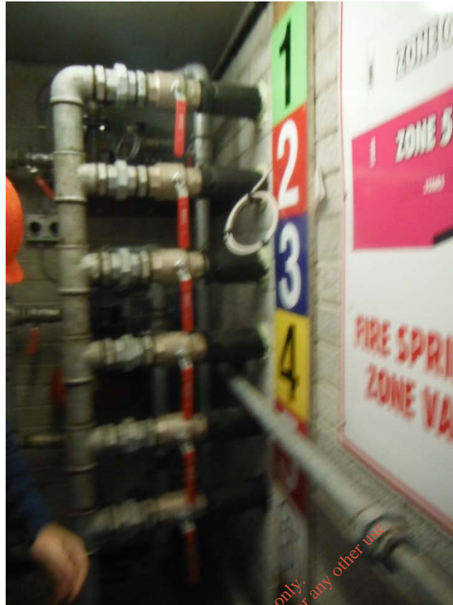
Figure 1.27: Pump House: Valves for Sprinkler System
