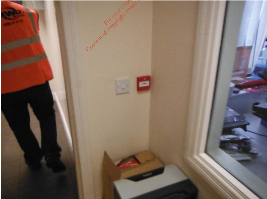
Figure 1.30: Office Building: Break Glass Alarm Unit
