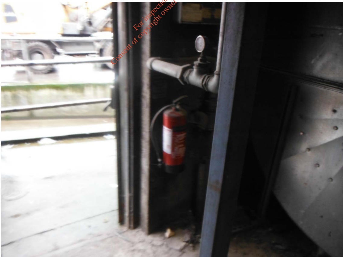
Figure 1.20: MRF: Fire Extinguisher by Exit
