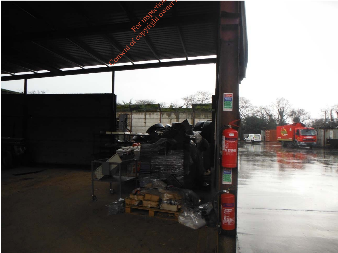
Figure 1.10: Plant Storage Shed: Fire Extinguisher at Entrance
