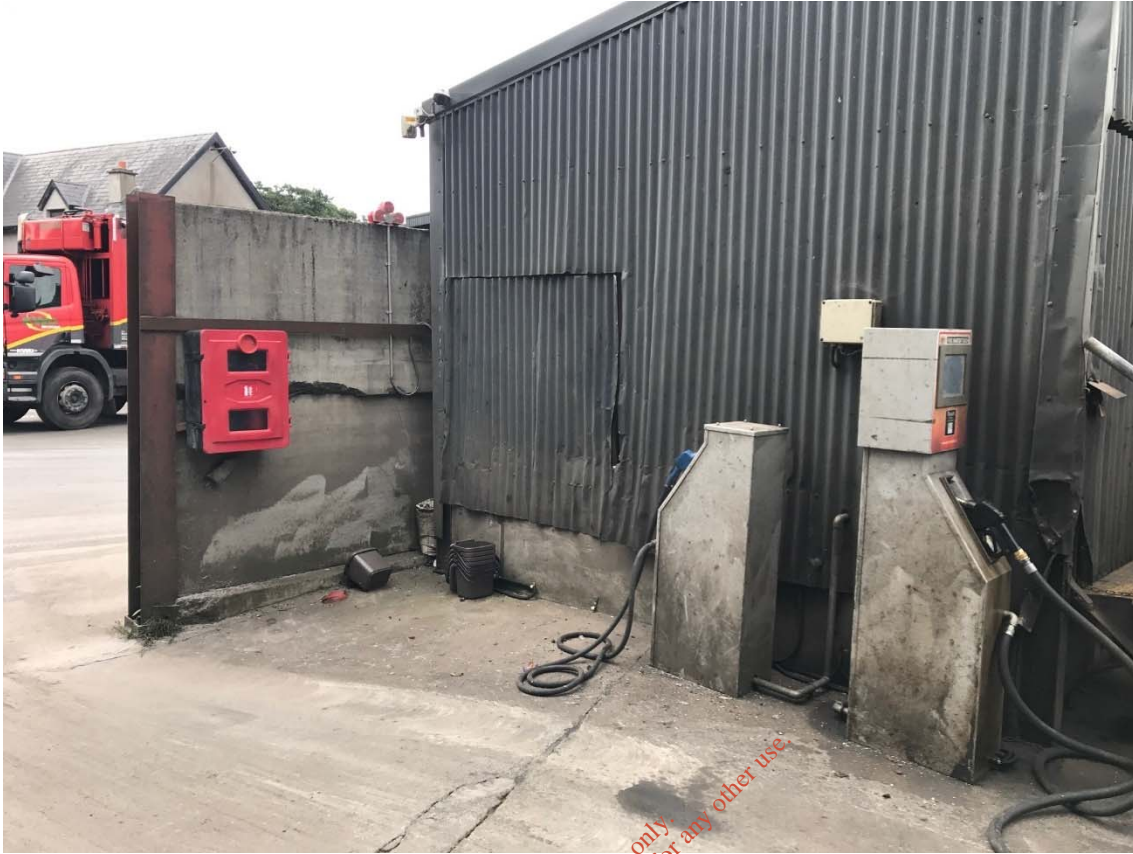
Figure 1.5: Yard Area: Diesel Pump and storage
