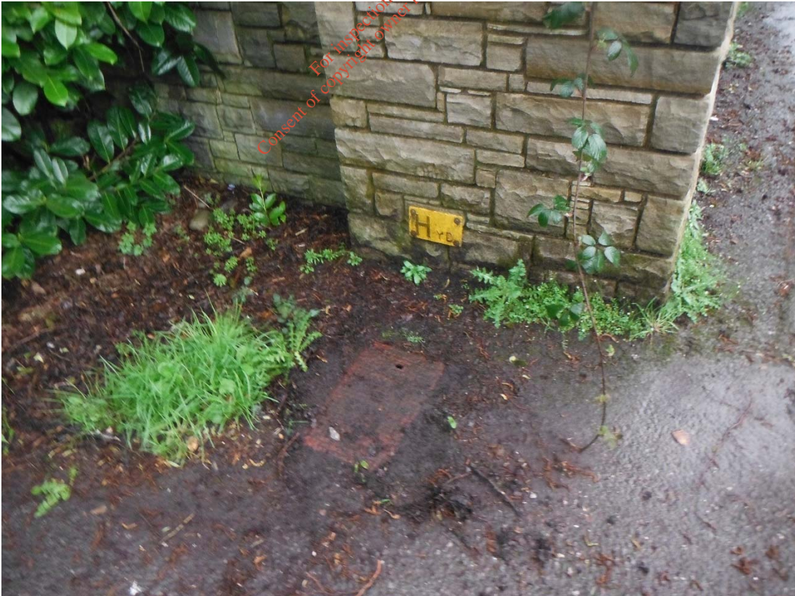
Figure 1.36: Road: Fire Hydrant by Entrance
