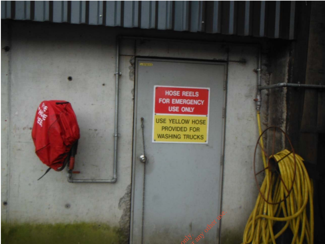
Figure 1.13: MRF: Fire Reel by Emergency Exit
