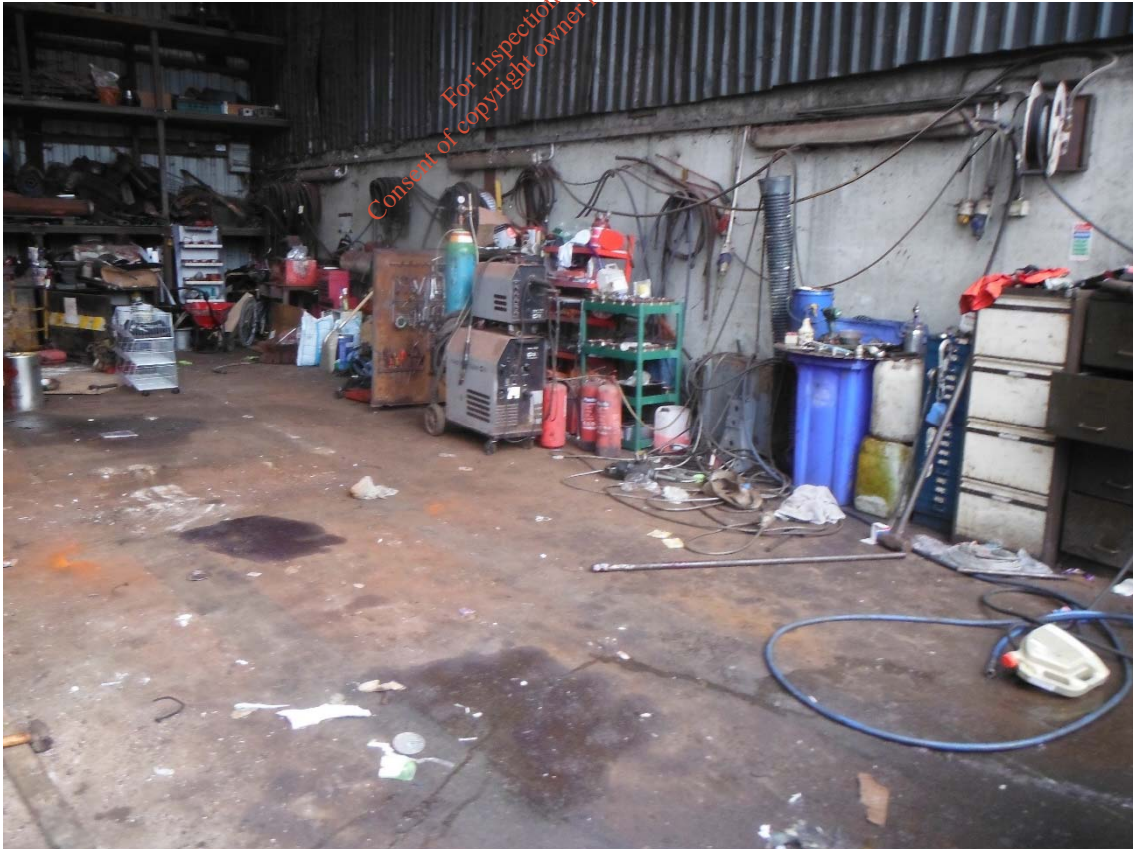
Figure 1.24: Workshop: Fire Extinguishers & Oxy Acetylene for Welding/Cutting
