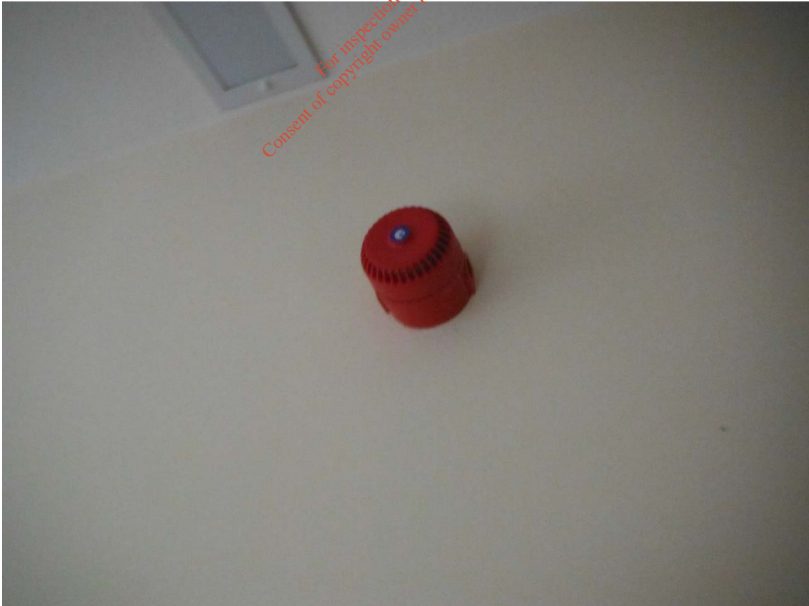
Figure 1.34: Office Building: Fire Alarm Beacon
