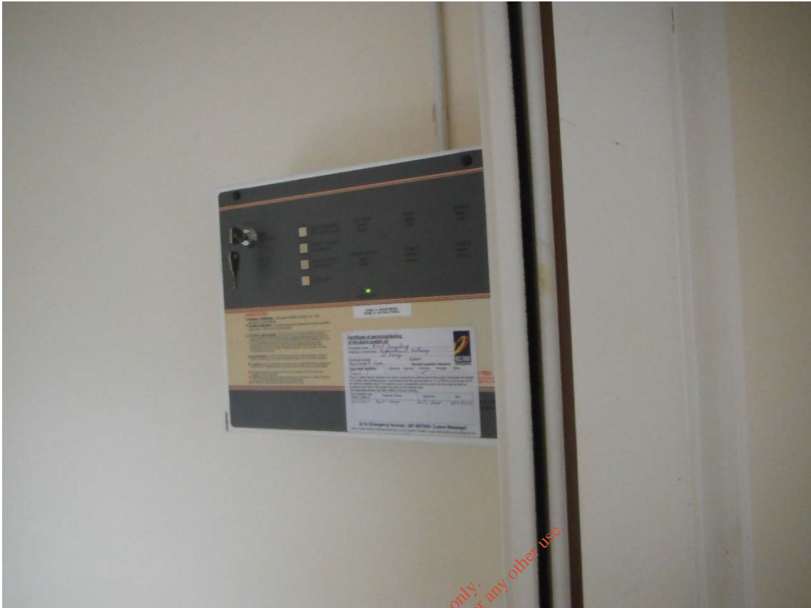
Figure 1.31: Office Building: Fire Alarm Control Box
