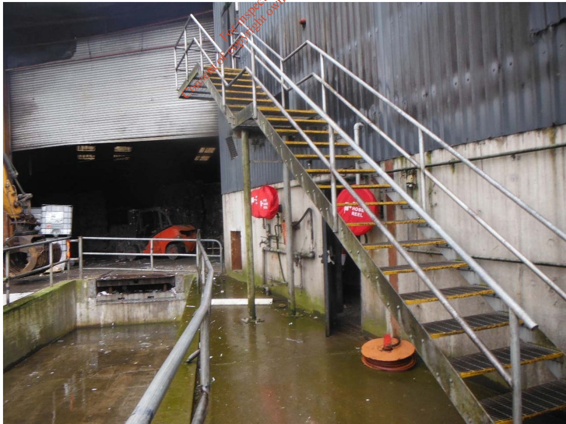
Figure 1.22: MRF: Fire Reels on West Side
