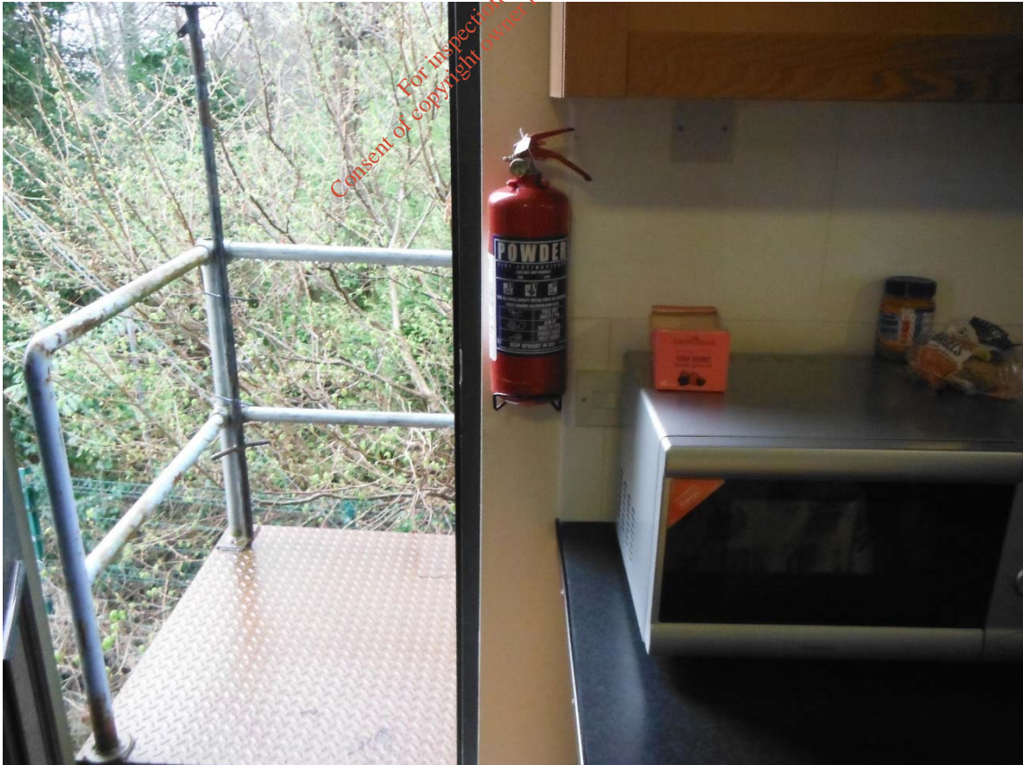
Figure 1.32: Office Building: Emergency Exit to Fire Stairs with Fire Extinguisher
