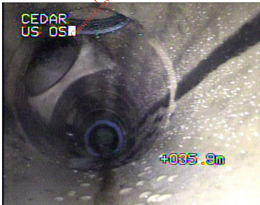
Photo: 52_8A, MPEG #: 051216_1, 00:05:26 36.1m, Connection other than junction, at 10 o'clock, diameter 100mm
