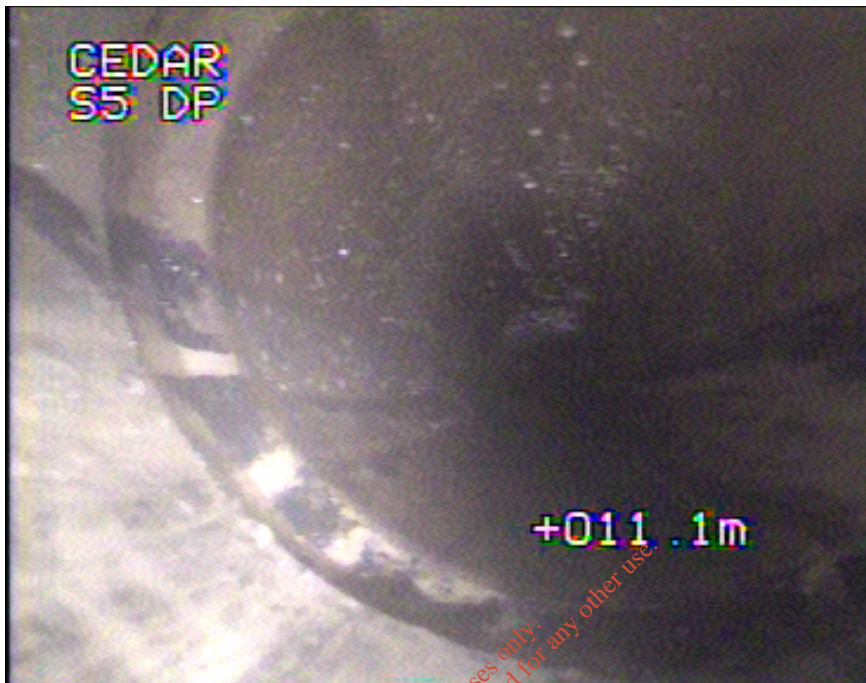
Photo: 27_9A, MPEG #: 051216_1, 00:01:44 11.1m, Open joint, medium
