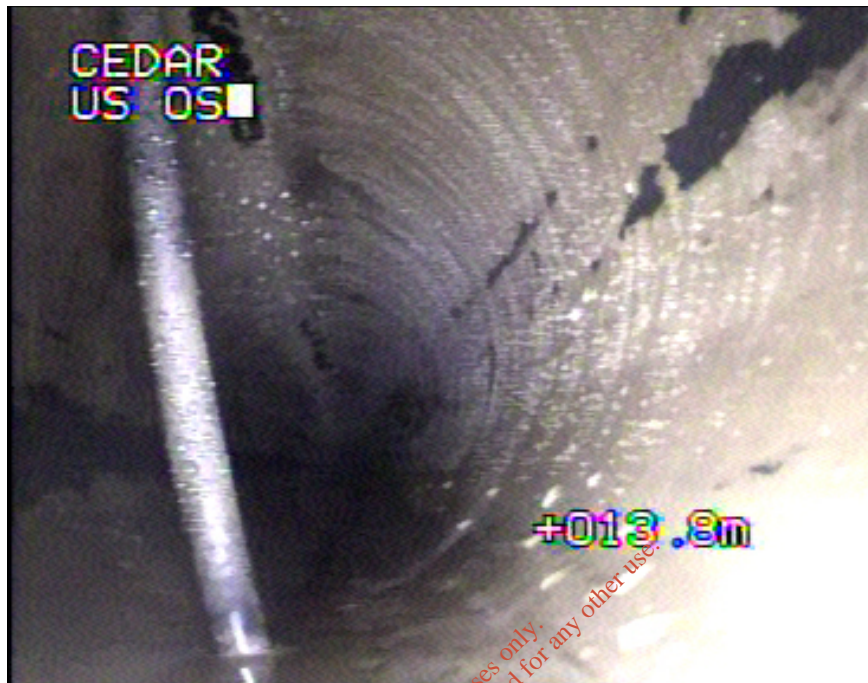
Photo: 52_3A, MPEG #: 051216_1, 00:01:52 14m, Other obstacles protruding through wall, from 12 to 6 o'clock, 5% cross-sectional area loss
