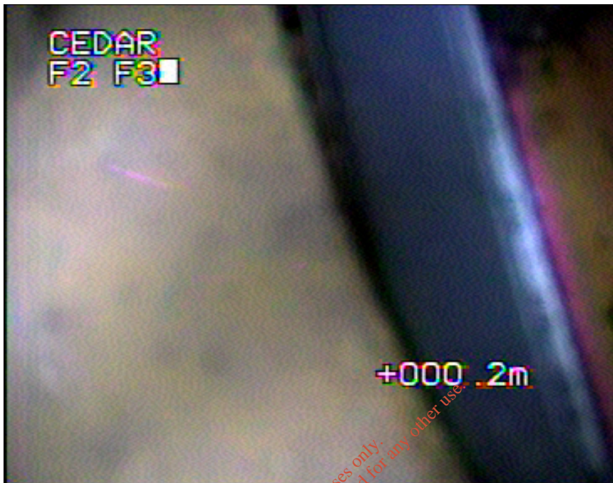
Photo: 4_3A, MPEG #: 051216_1, 00:00:07 0.2m, Sealing ring intruding, from 6 to 12 o'clock
