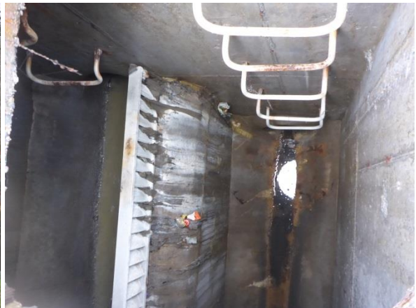
Image 4: Mains on left with screen on overflow
