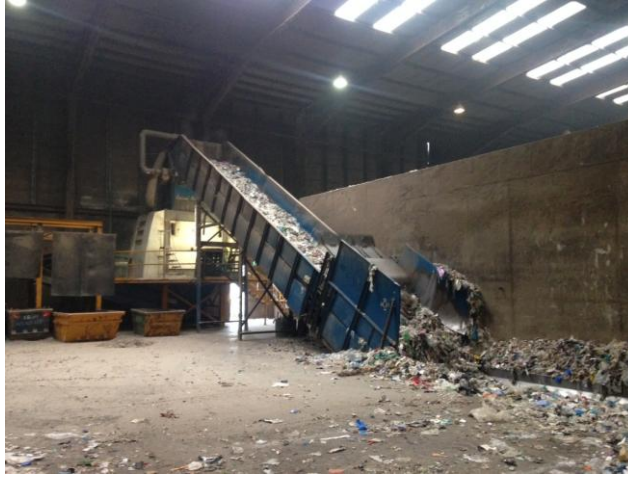
Intake for solid recovered fuel production facility (Untha 2) in Building 2
