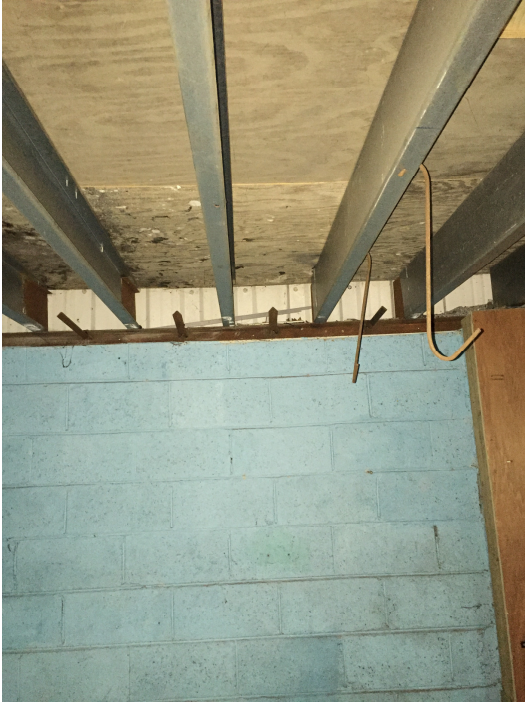
Figure 13: No Fire Detection and Alarm System
