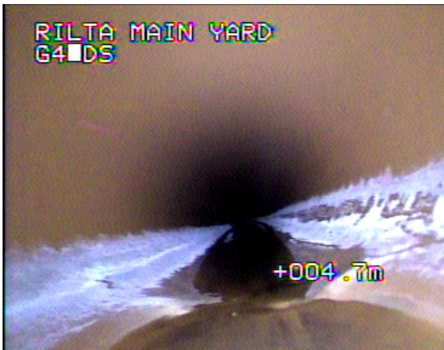
Photo: 38_5A, MPEG #: 280217_1, 00:00:33 4.7m, Surface damage, other, from 4 to 8 o'clock
