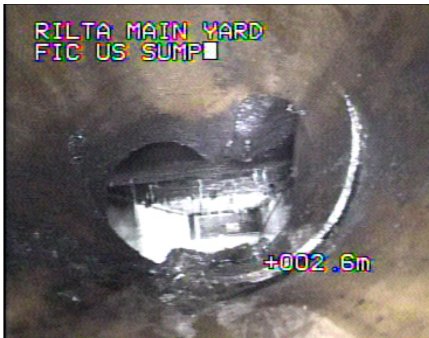
Photo: 19_4A, MPEG #: 280217_1, 00:00:51 2.8m, Fracture, circumferential, from 2 to 7 o'clock
