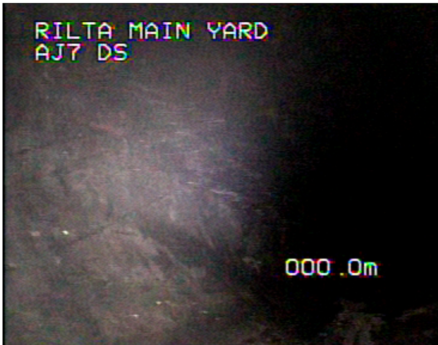
Photo: 45_9A, MPEG #: 280217_1, 00:00:00 39.59m, Other obstacles built into structure, from 1 to 3 o'clock, 75% cross-sectional area loss
