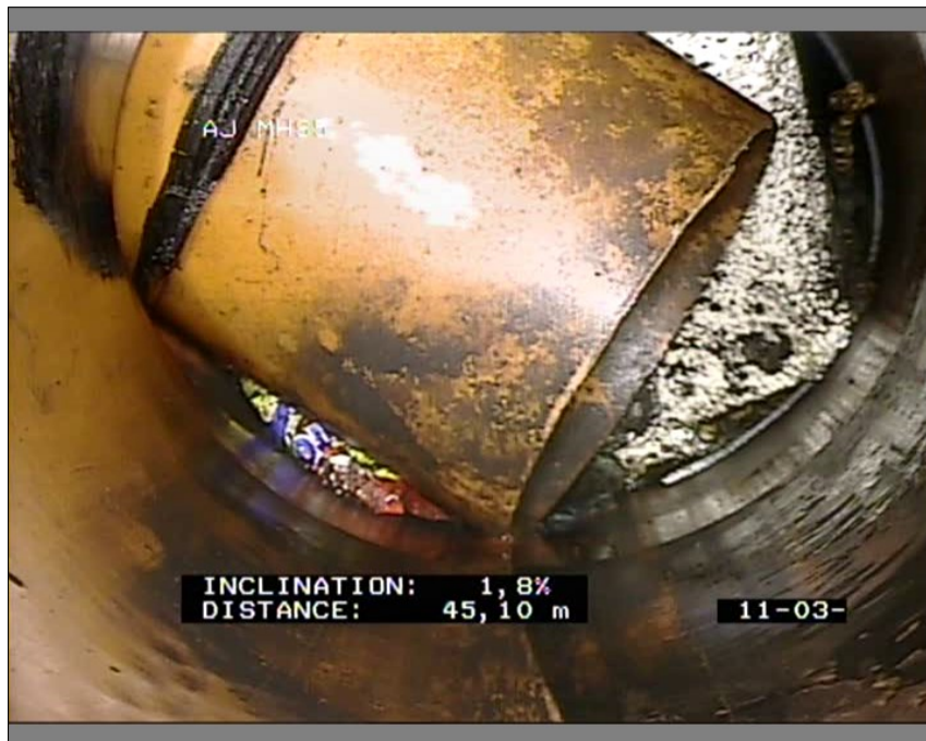
Photo: 8_14A, MPEG #: 280217_1, 00:13:29 45.49m, Connection other than junction, at 10 o'clock, diameter 100mm
