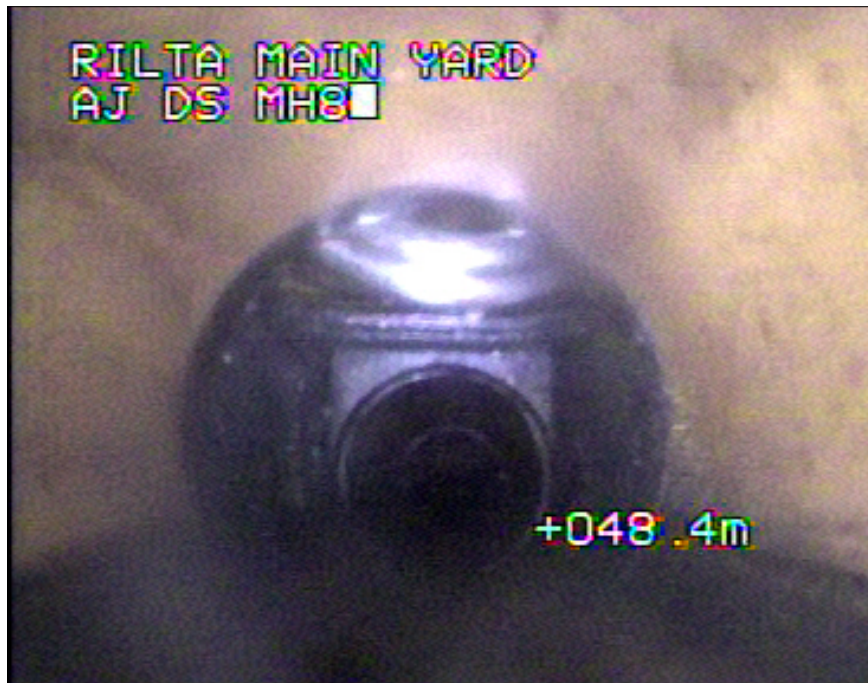
Photo: 53_17A, MPEG #: 280217_1, 00:07:29 48.5m, Sealing ring intruding, from 11 to 2 o'clock
