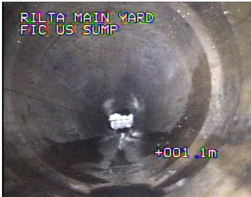
Photo: 19_3A, MPEG #: 280217_1, 00:00:27 1.1m, Open joint, medium
