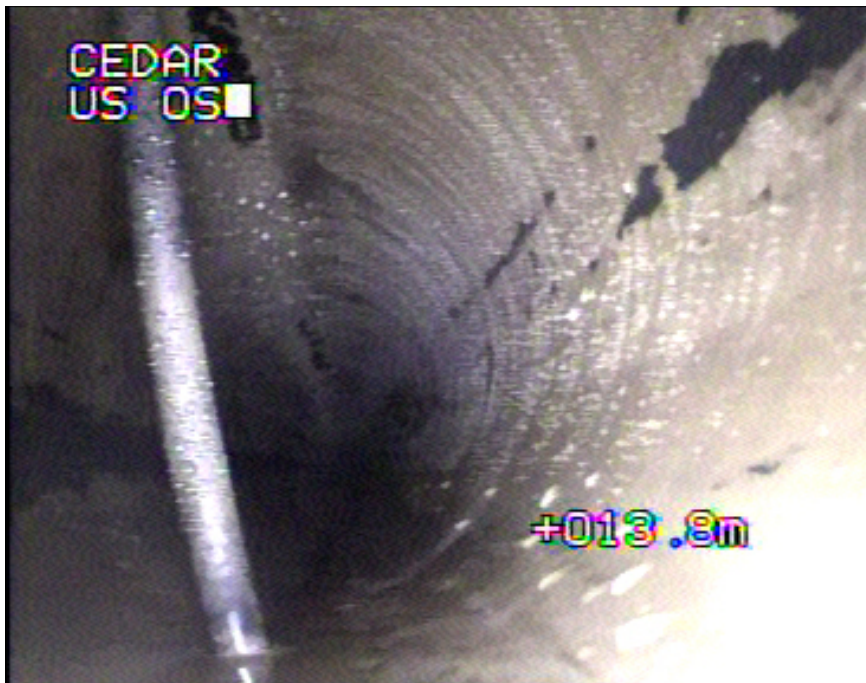
Photo: 52_3A, MPEG #: 051216_1, 00:01:52 14m, Other obstacles protuding through wall, from 12 to 6 o'clock, 5% cross-sectional area loss
