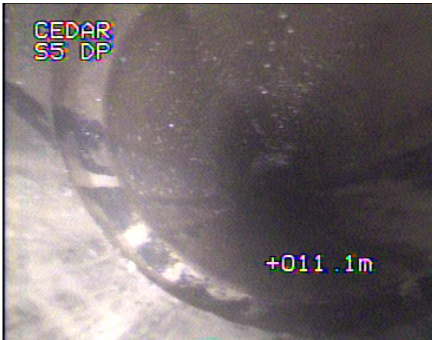
Photo: 27_9A, MPEG #: 051216_1, 00:01:44 11.1m, Open joint, medium
