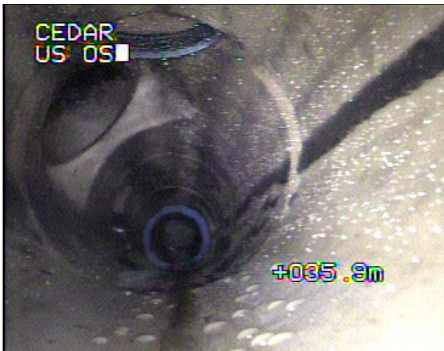
Photo: 52_8A, MPEG #: 051216_1, 00:05:26 36.1m, Connection other than junction, at 10 o'clock, diameter 100mm
