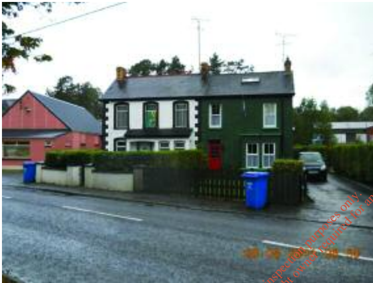
Green house (98 Avenue) flooded to a depth of four inches in November 2009
