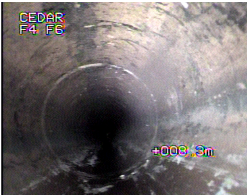
Photo: 7_5A, MPEG #: 051216_1, 00:01:22 8.3m, Cracks, multiple, from 4 to 8 o'clock
