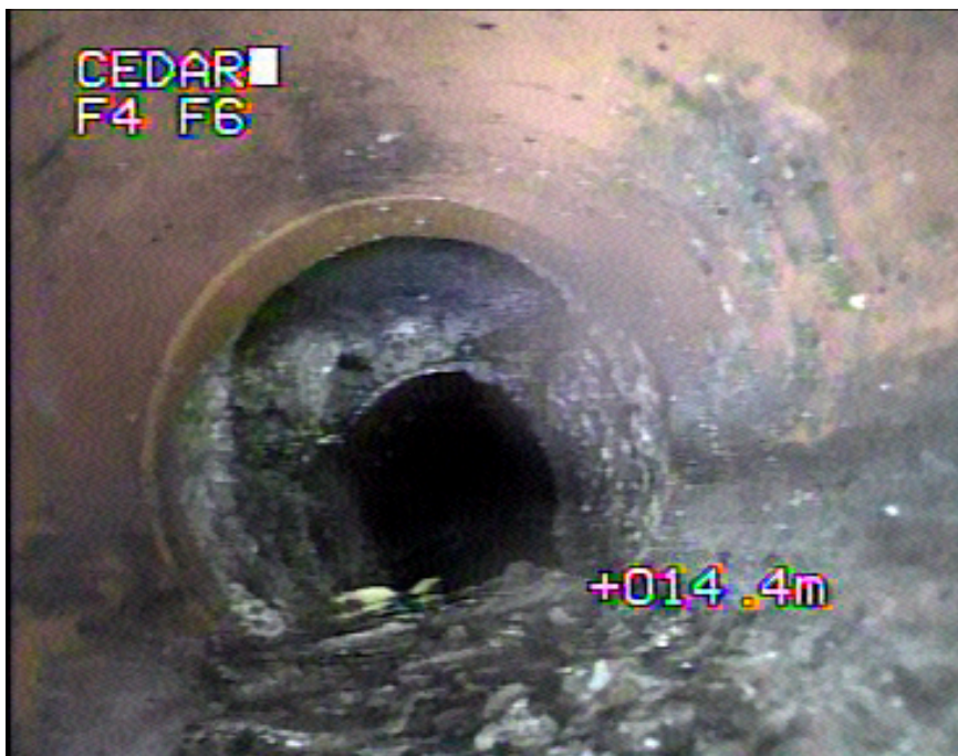
Photo: 7_6A, MPEG #: 051216_1, 00:02:24 14.3m, Settled deposits, hard or compacted, 10% cross-sectional area loss
