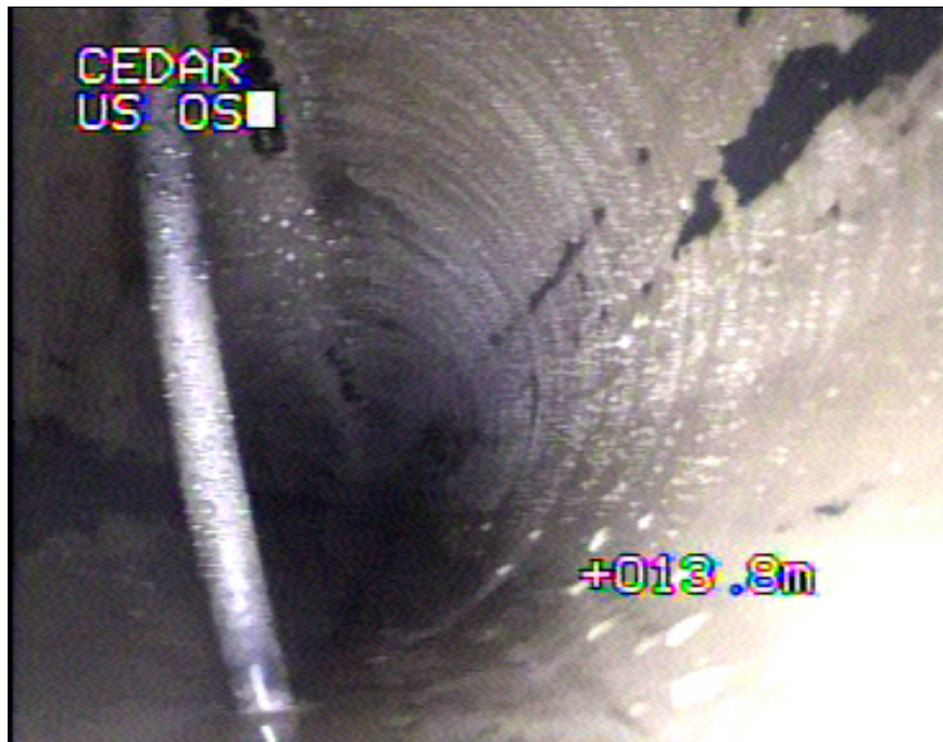
Photo: 52_3A, MPEG #: 051216_1, 00:01:52 14m, Other obstacles protuding through wall, from 12 to 6 o'clock, 5% cross-sectional area loss
