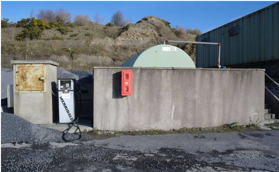
Photo 1 - Bunded 70,000 litre Diesel Tank
