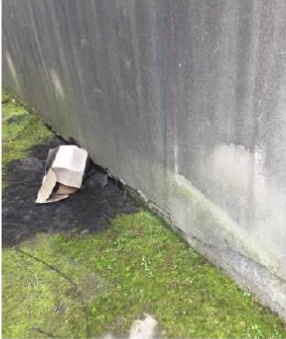
Figure 2-2 Leak from base of bund wall
