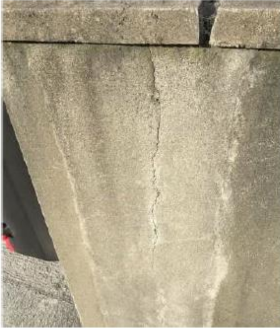
Figure 2-1 Example of crack in bund wall
