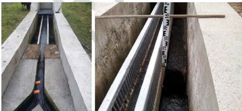
Fig 4.2 – Storm Overflow at WWTP
