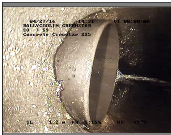
Photo: 14_14_65_A.JPG 1.28m, Connection intruding, at 12 o'clock, diameter 150mm, intrusion 20%
