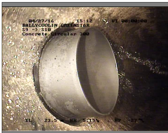
Photo: 16_16_83_A.JPG 23.52m, Connection intruding, at 11 o'clock, diameter 150mm, intrusion 30%
