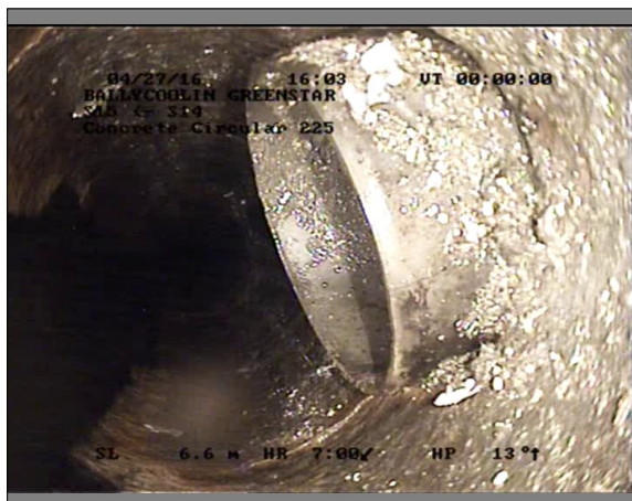
Photo: 18_18_93_A.JPG 6.65m, Connection intruding, at 12 o'clock, diameter 150mm, intrusion 30%
