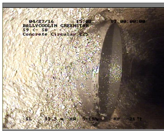
Photo: 15_15_76_A.JPG 33.5m, Connection intruding, at 12 o'clock, diameter 150mm, intrusion 15%
