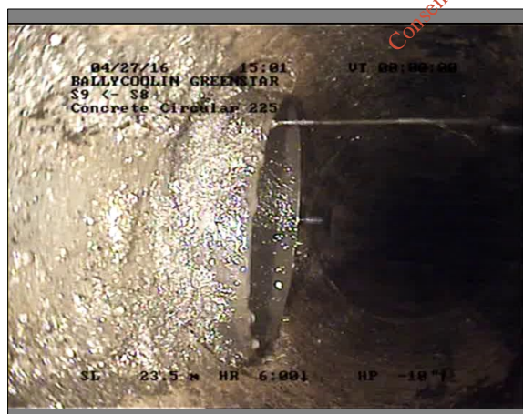
Photo: 15_15_74_A.JPG 23.5m, Connection intruding, at 12 o'clock, diameter 150mm, intrusion 15%
