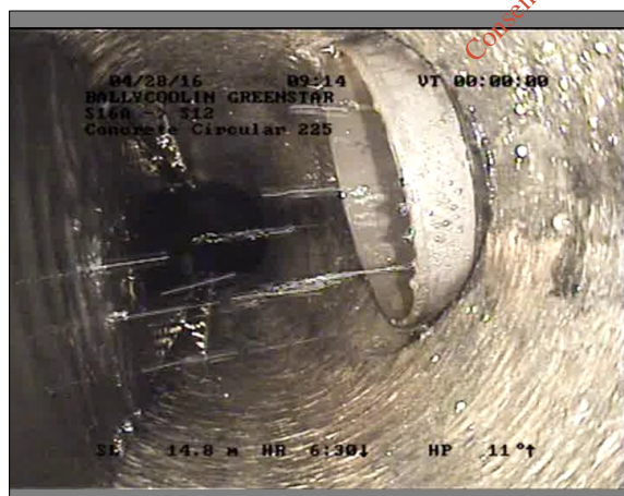
Photo: 22_22_117_A.JPG 14.81m, Connection intruding, at 12 o'clock, diameter 150mm, intrusion 15%
