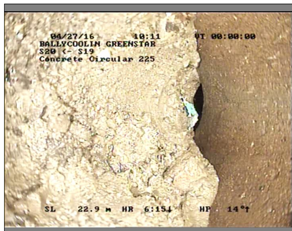
Photo: 3_3_6_A.JPG 22.93m, Settled deposits, hard or compacted, 95% cross-sectional area loss Remarks: Concrete
