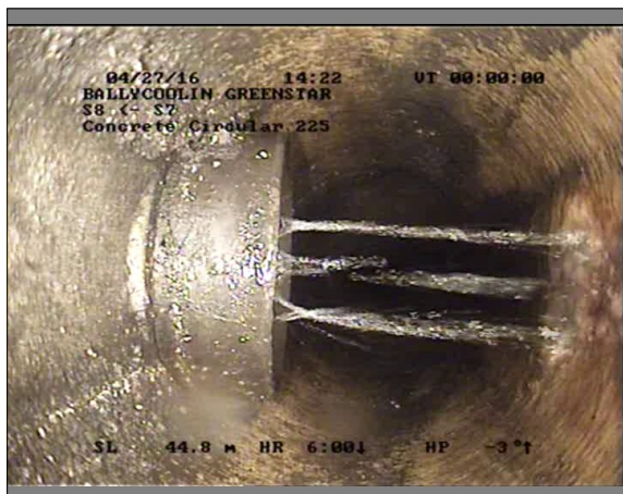
Photo: 13_13_61_A.JPG 44.81m, Connection intruding, at 12 o'clock, diameter 150mm, intrusion 20%
