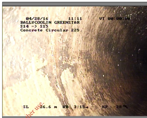
Photo: 23_23_127_A.JPG 26.67m, Fracture, circumferential, from 7 to 11 o'clock
