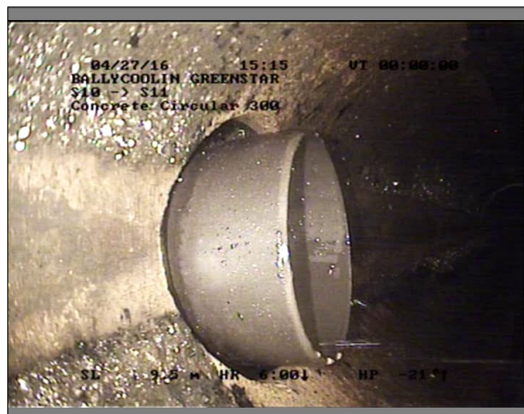
Photo: 17_17_87_A.JPG 9.57m, Connection intruding, at 12 o'clock, diameter 150mm, intrusion 30%
