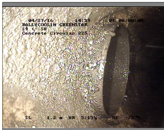
Photo: 15_15_71_A.JPG 1.2m, Connection intruding, at 12 o'clock, diameter 150mm, intrusion 15%
