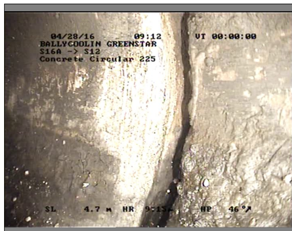
Photo: 22_22_114_A.JPG 4.74m, Open joint, 5mm of diameter
