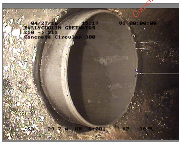
Photo: 17_17_89_A.JPG 29.75m, Connection intruding, at 12 o'clock, diameter 150mm, intrusion 15%
