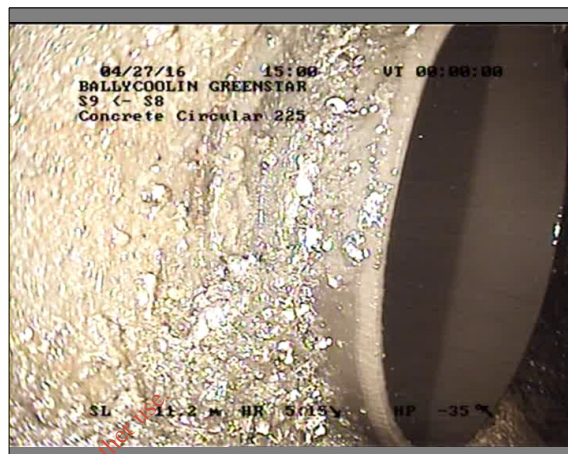
Photo: 15_15_73_A.JPG 11.2m, Connection intruding, at 12 o'clock, diameter 150mm, intrusion 15%
