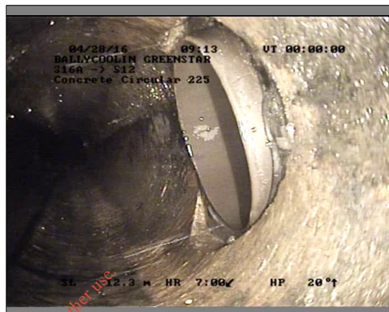
Photo: 22_22_115_A.JPG 12.33m, Connection intruding, at 12 o'clock, diameter 150mm, intrusion 10%
