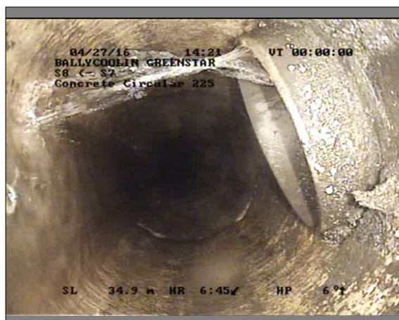
Photo: 13_13_59_A.JPG 34.94m, Connection intruding, at 12 o'clock, diameter 150mm, intrusion 20%
