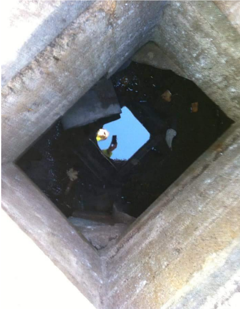
FIGURE 1: SURFACE WATER DRAIN CONNECTED TO SWO-NO FLOW ON ASSESSMENT DAY
