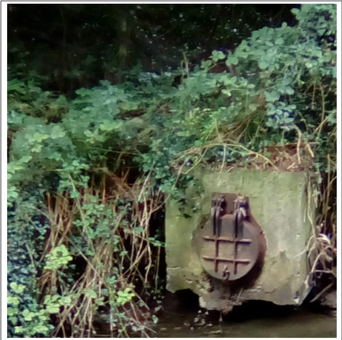
Figure 1: Storm water overflow pipe at Deerpark pumping station:
