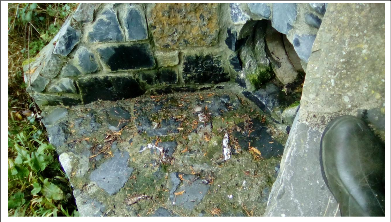
FIGURE 1: STORM WATER OVERFLOW AT RATOATH PUMPING STATION:
