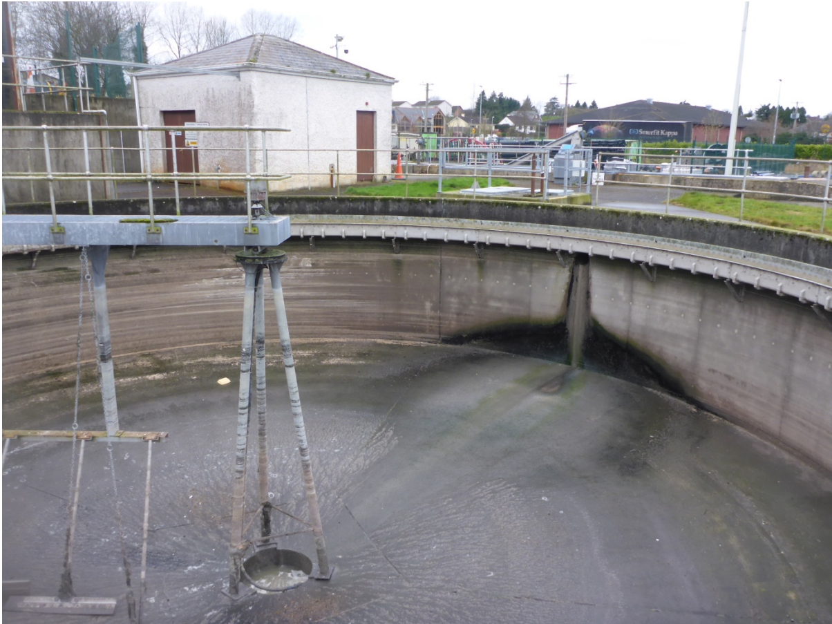
Photo 2 – 450m 3 storm water holding tank
