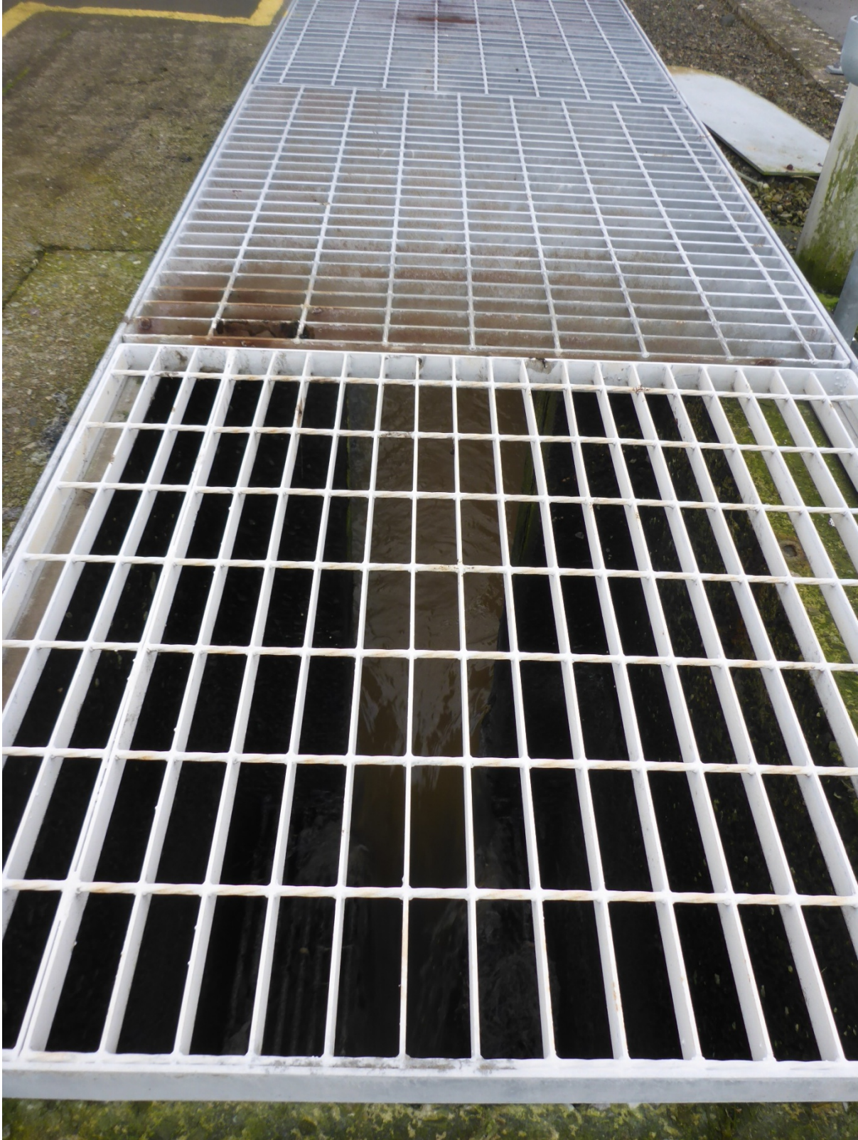
Photo 1 – SW-2 at the inlet works.
