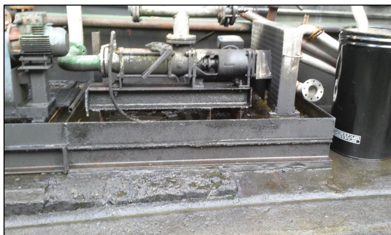
Figure 11 Evidence of improved yard and bund cleaning (October 2016)
