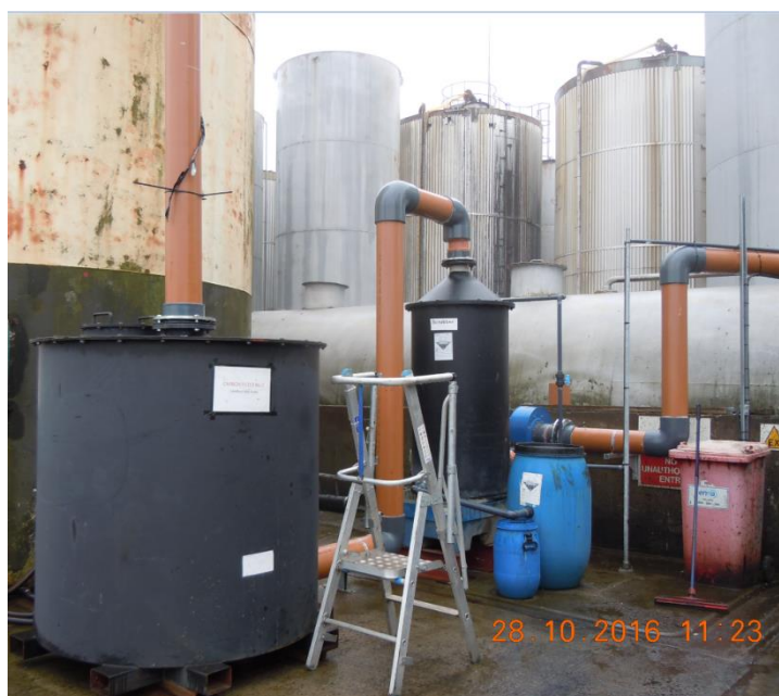
Figure 16 Acid scrubber (taller black tank in centre) and carbon filter (shorter black tank on left) for treatment of mechanically-drawn off-gas emissions from the Hodgefield oil-water separator
