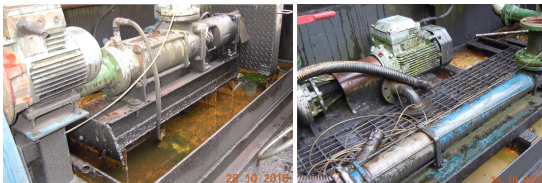
Figure 17 Bunds that require cleaning
