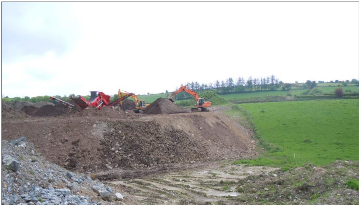
Figure 4 Photo taken on 16 th May 2016 showing a bank some 5 to 6 metres high
