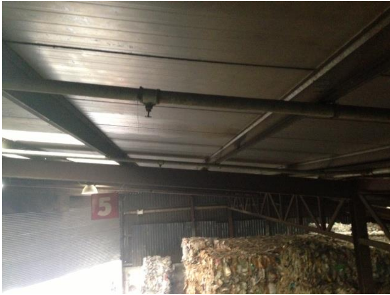
Pipe Work and Sprinkler Heads
