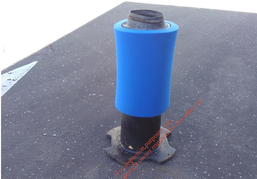
Photo D.1.5 – New Filter on Foul Line Interceptor
