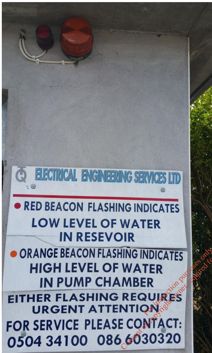
Photo D.1.8 – Notice on site Detailing Alarms in Balancing Tank
