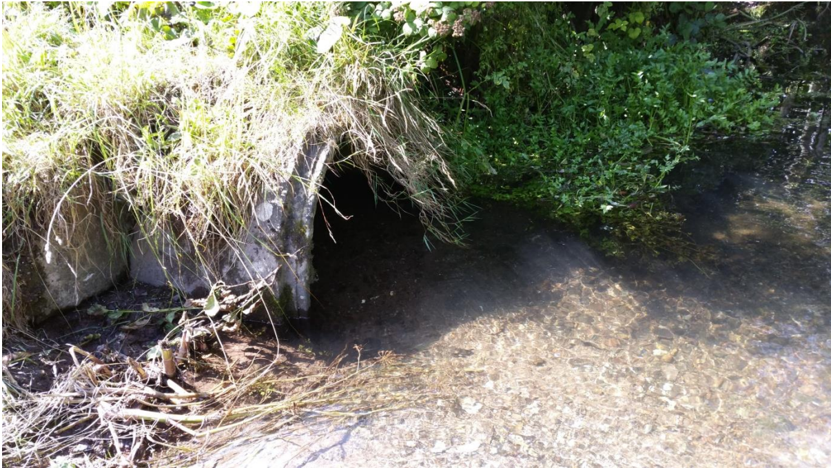
Photo D.1.10 – Discharge of Culverted Local Stream into Tramore River (370 north of site)
