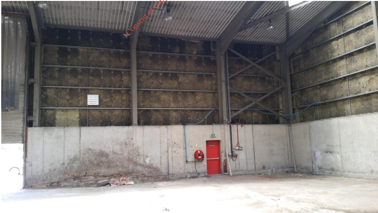
Photo D.1.13 – Acoustic Insulation in Building 2.
