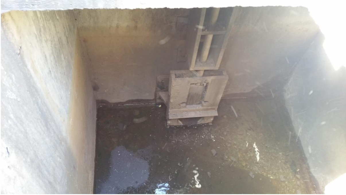
Photo D.1.7 – Manual Shut-Off Valve at Stormwater Discharge Point (SW1)
