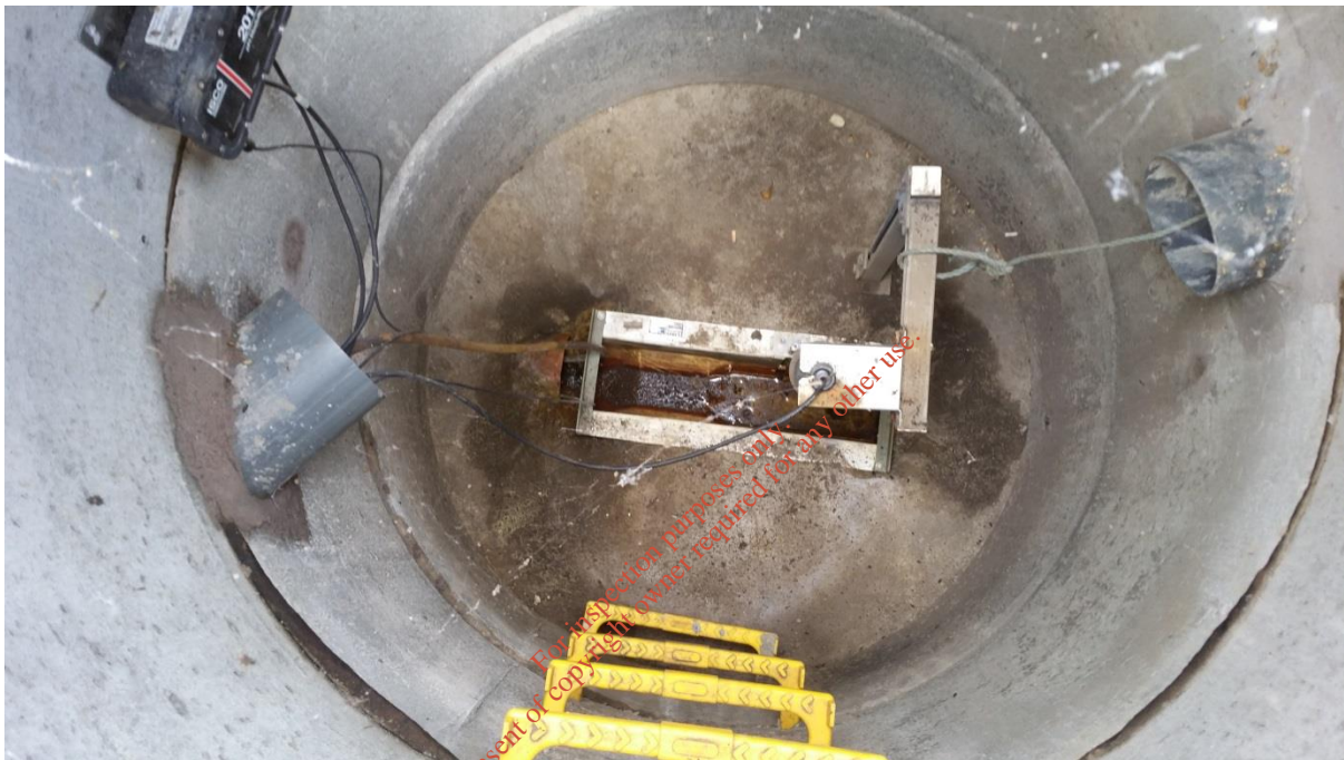
Photo D.1.4 – Monitoring Equipment on the Sewer Line
