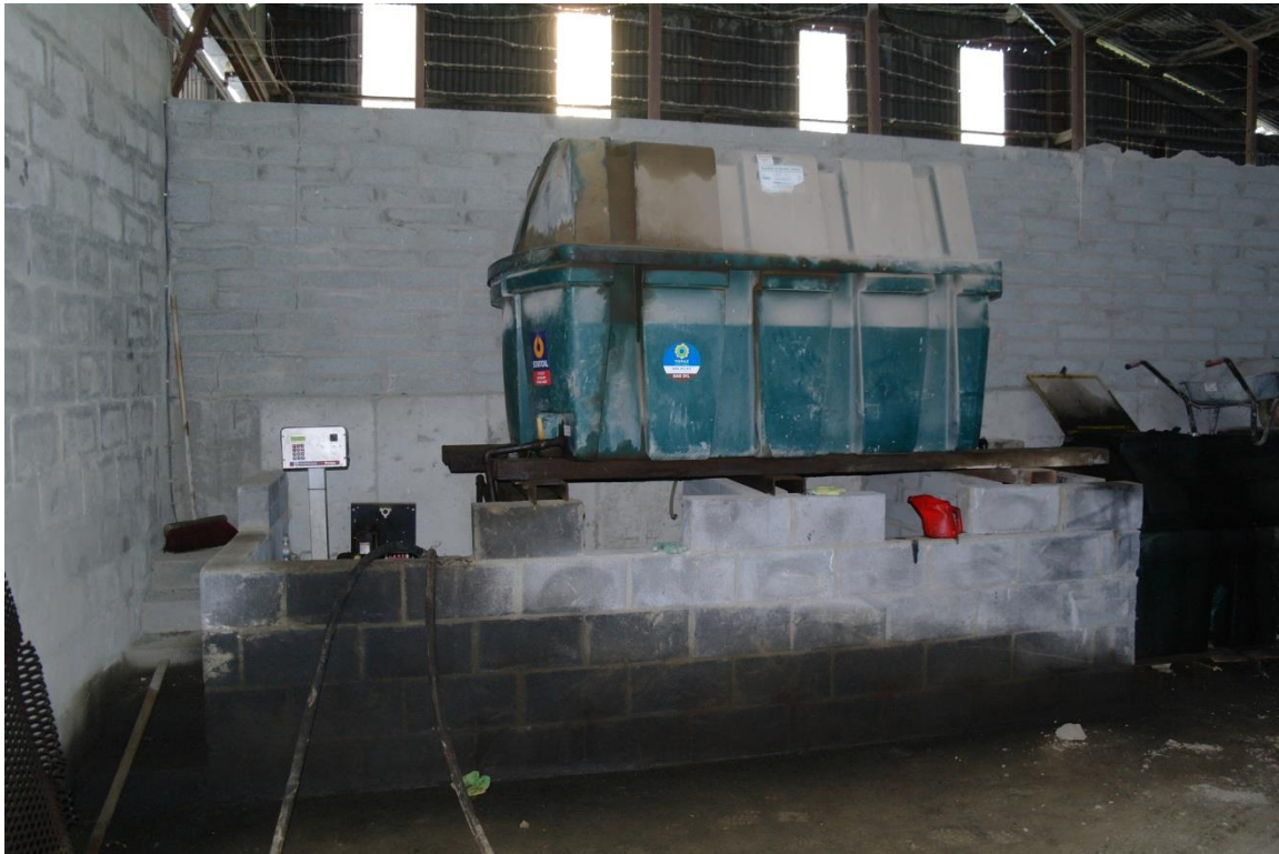
Photo 3 – Bunded Gas Oil (Diesel) Tank in Maintenance Shed
