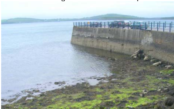
15. View looking WNW out to the old pier. A series of recesses in the upper tier of concrete are putlog holes that may have supported a boardwalk feature.
