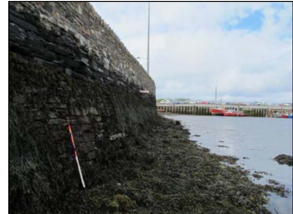
24. Looking W along base of south quay showing the slightly battered or sloped nature of the walling and the shingle covered shore which has some fallen stonework.
