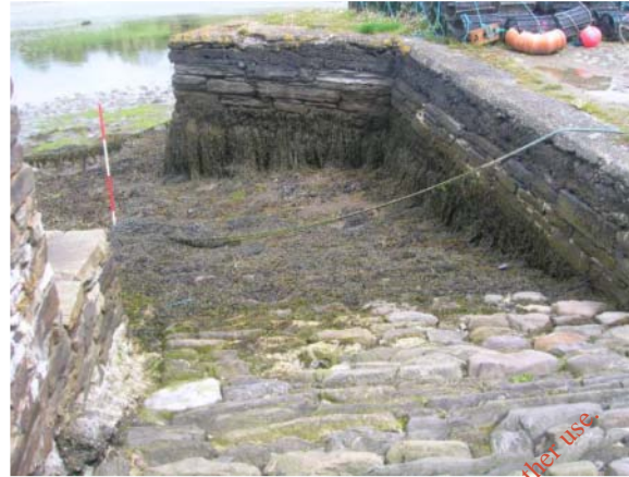
Slip showing original stonework on east side, and reconstructed stonework on left (west) side
