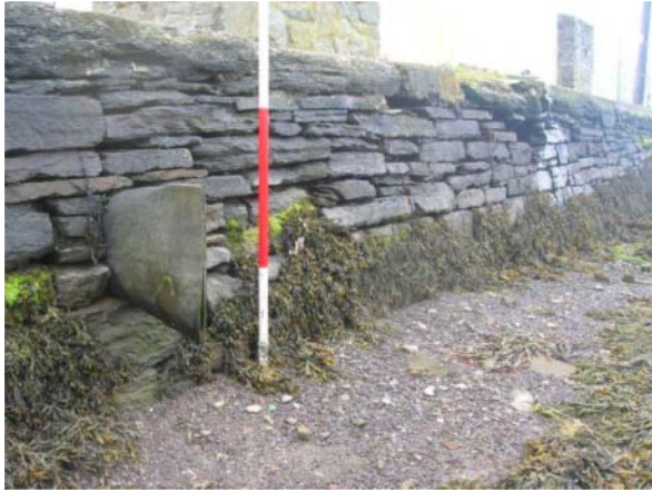
22. View looking W along south quay, highlighting a modern outfall fitted with a rubberized valve (ADCO 12) integrated into the traditional stone build.
