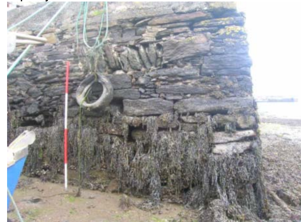
Detail showing straight-wall return of west side slip, including a relieving-arch feature
