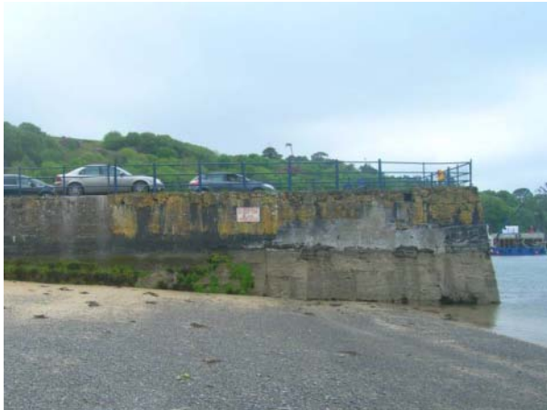
12. Pier Head from North. Notice build line in concrete indicating the extension of the pier.
