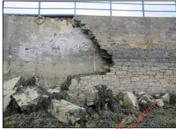
13. Looking N showing the ruinous nature of the stone façade to the concrete pier head.
