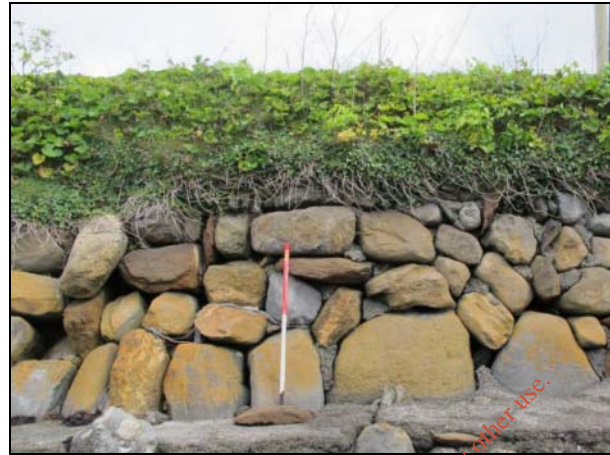
17. View looking at alternative blockier stonework forming the modern revetment along the north shore
