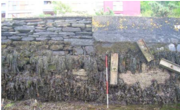
25. View of south quay where the stonework of the old quay is replaced with poured concrete work, marking the extension of the quay.
