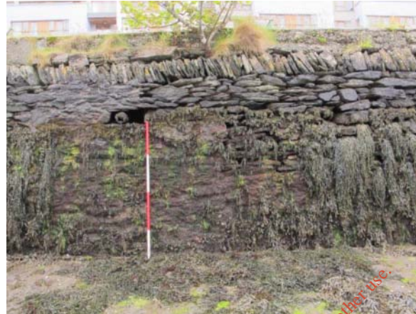
23. View of south quay west of the third slipway (ADCO 21), showing the worn nature of the stonework in the upper levels, and an upper course of edge-set stone. The top surface has been capped with concrete.
