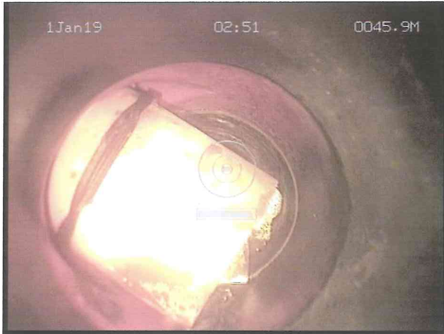
Photo: 14_5a 46.2m, Connection defective, at 10 o'clock, dia 125 mm, intrusion 200 mm
