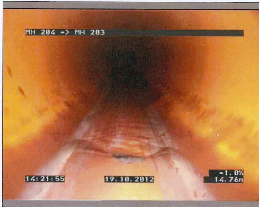
Photo: 1_3A, MPEG #: 311013_1, 00:03:07 14.76m, Deformed sewer, 5% of original diameter/height
