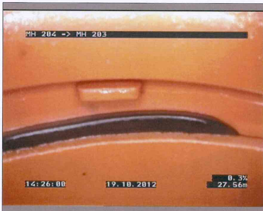
Photo: 1_4A, MPEG #: 311013_1, 00:06:31 27.49m, Open joint, medium (between 1.0 and 1.5 times the pipe wall thickness)
