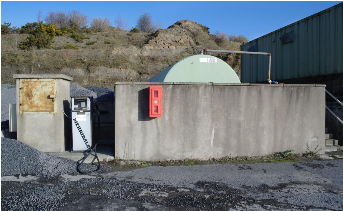
Photo 1 - Bunded 70,000 litre Diesel Tank
