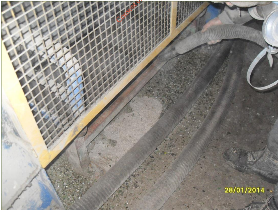
Photograph F.1.8: Industrial vacuum system spot cleaning hose in Drying Plant (2)
