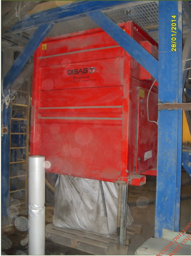
Photograph F.1.7: Industrial vacuum system in Drying Plant (1)
