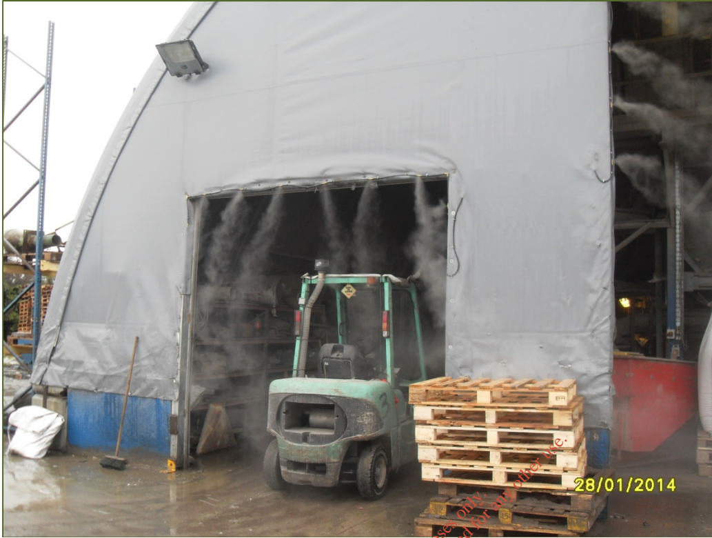
Photograph F.1.5: Misting system at Drying Plant (3)
