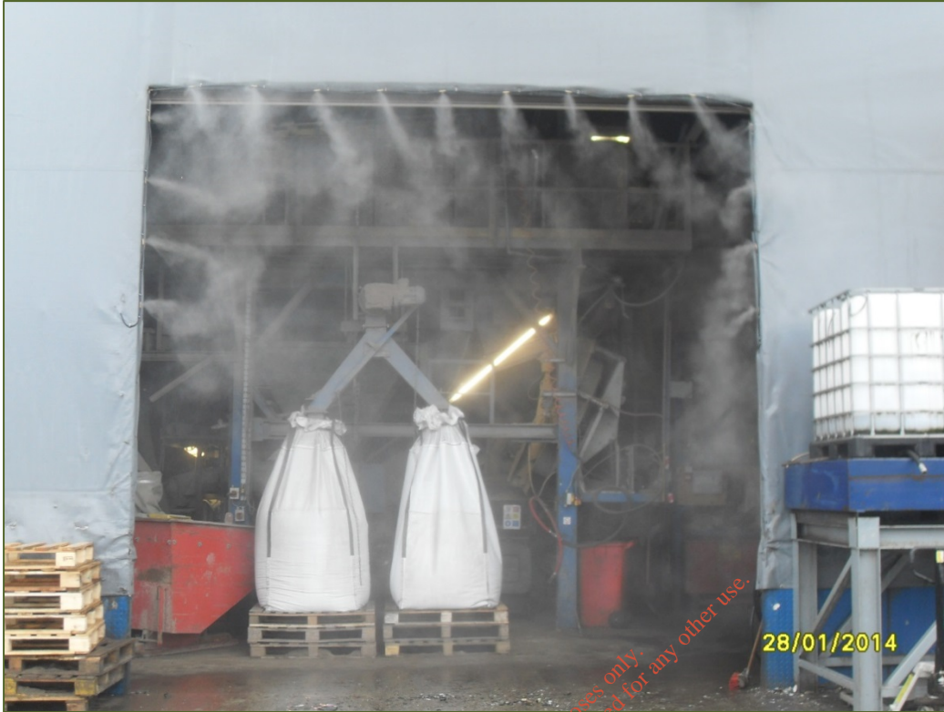
Photograph F.1.3: Misting system at Drying Plant (1)
