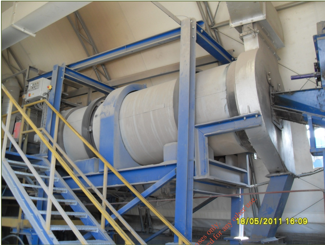
Photograph D.1.7: Rotating Drying Unit (Drying Plant building)
