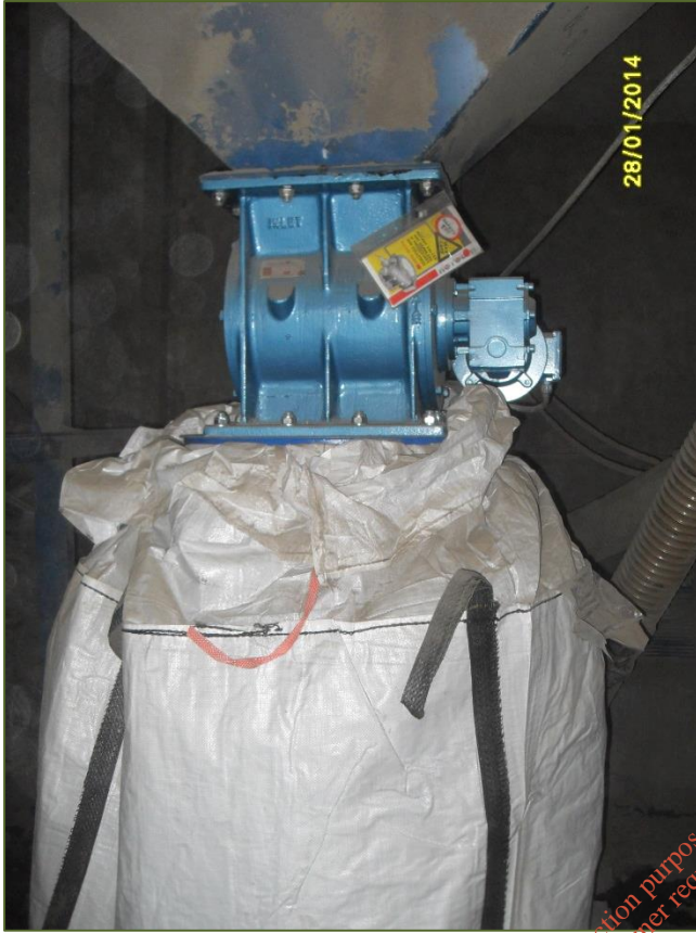
Photograph F.1.9: Sealed/contained chutes/silos to storage bags in Drying Plant (2)
