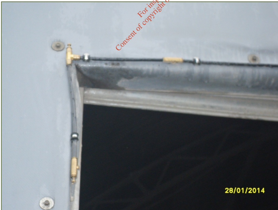
Photograph F.1.6: Misting system at Drying Plant (4) – spray nozzles
