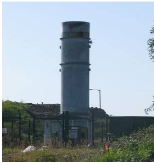
Figure 3.10: Enclosed Landfill Gas Flare at Powerstown landfill
