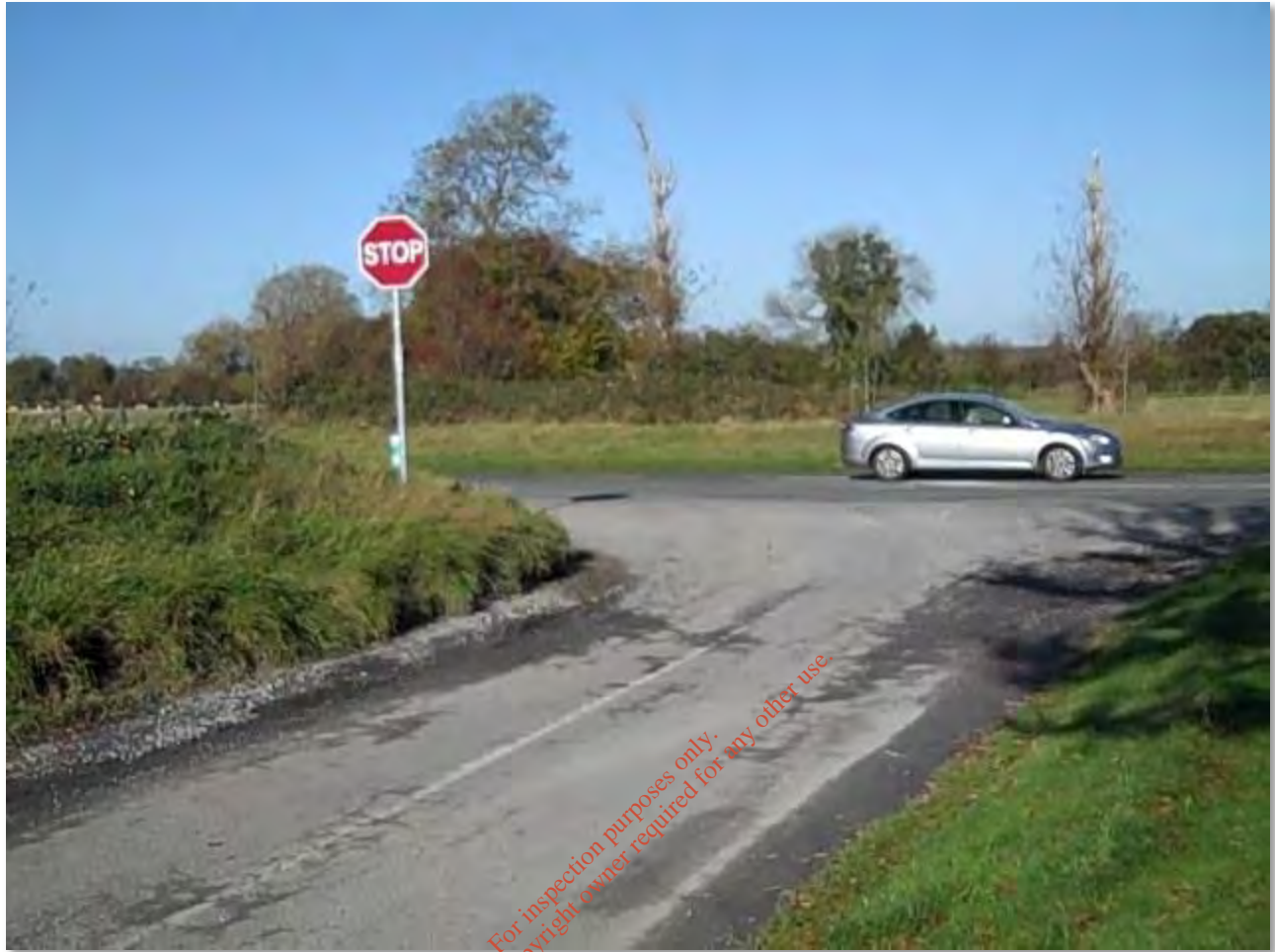
Figure 2.7 Rutting, cracking and edge deterioration on Jock's Lane at N80 junction
