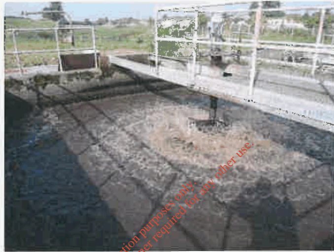
PHOTO: AERATION TANK AT KILFENORA WWTP
