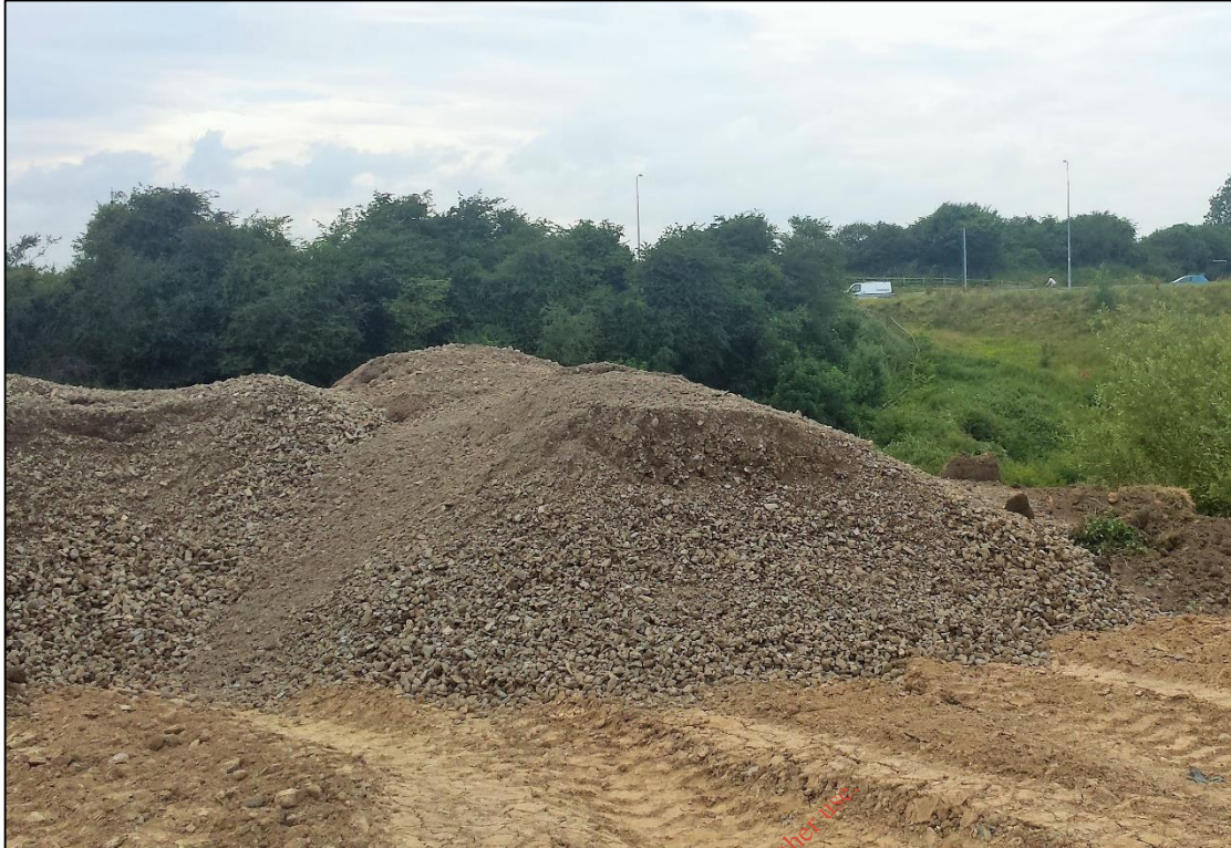
View 1: Restoration Works within Grannagh Site looking NW towards the new N24
