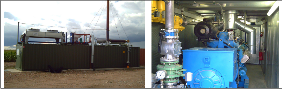
Figure 8 Containerised CHP at the Decker biogas plant in Northern Germany
