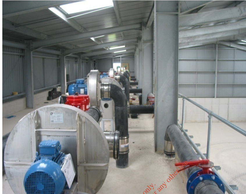
Figure 11 The blower modules in the gallery of the Deepmoor tunnel composting facility in Devon
