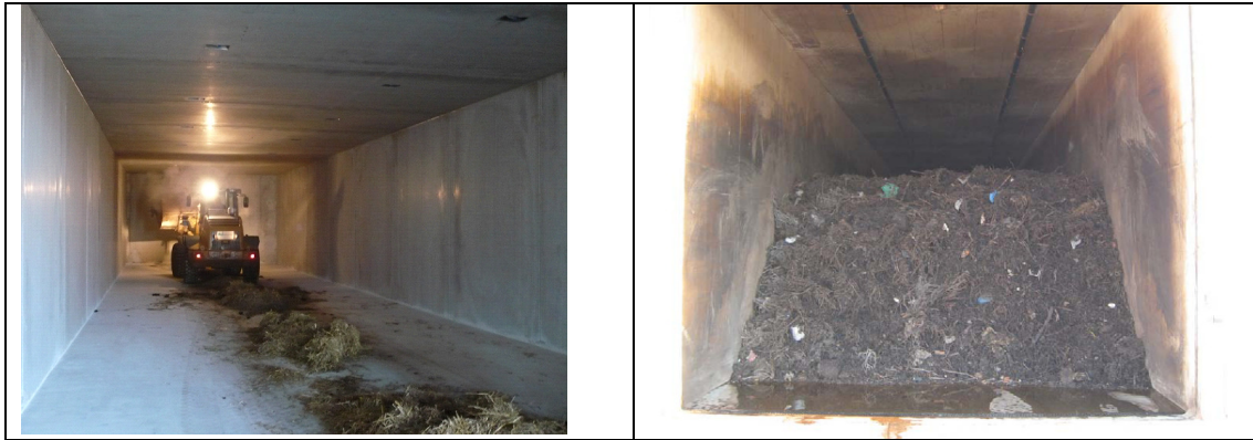
Figure 6 Interior of fermenter prior to filling (left) and with bio-waste prior to fermenter sealing.
