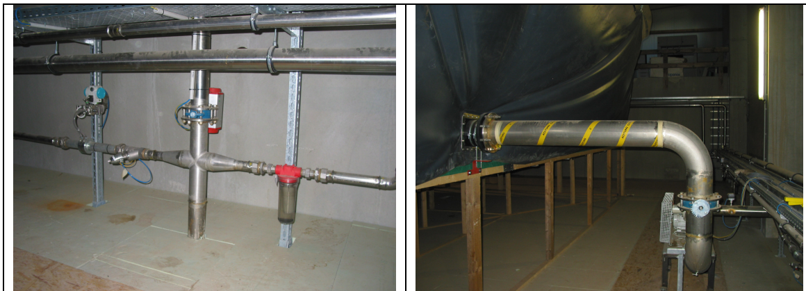
Figure 7 The pneumatic gas collection system on the roof of the fermenters (left) and the gas transfer blower to the gas bag (right).
