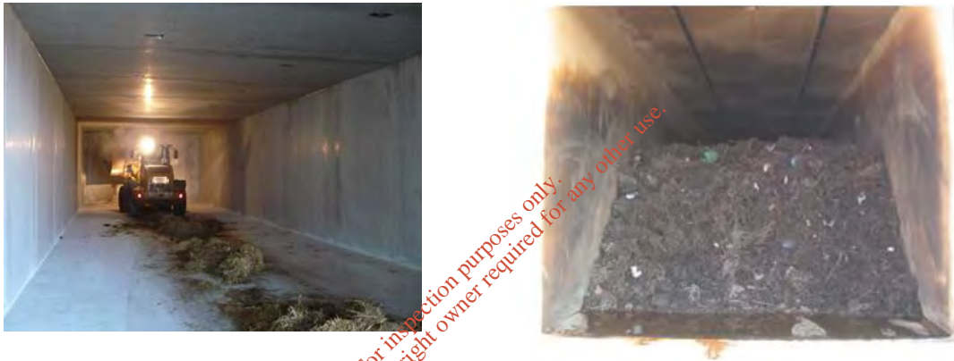
Fig. 4. Interior of fermenter prior to filling (left) and with bio-waste prior to fermenter sealing.
