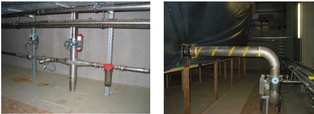
Fig. 8. The pneumatic gas collection system on the roof of the fermenters (left) and the gas transfer blower to the gas bag (right).
