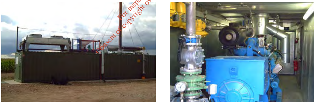
Fig.9. Containerised CHP at the Decker biogas plant in Northern Germany
