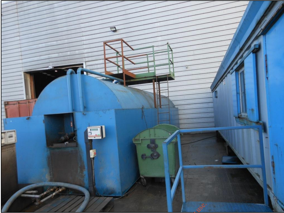
Photo 1 Locus of the steel oil bund and tank at the facility
