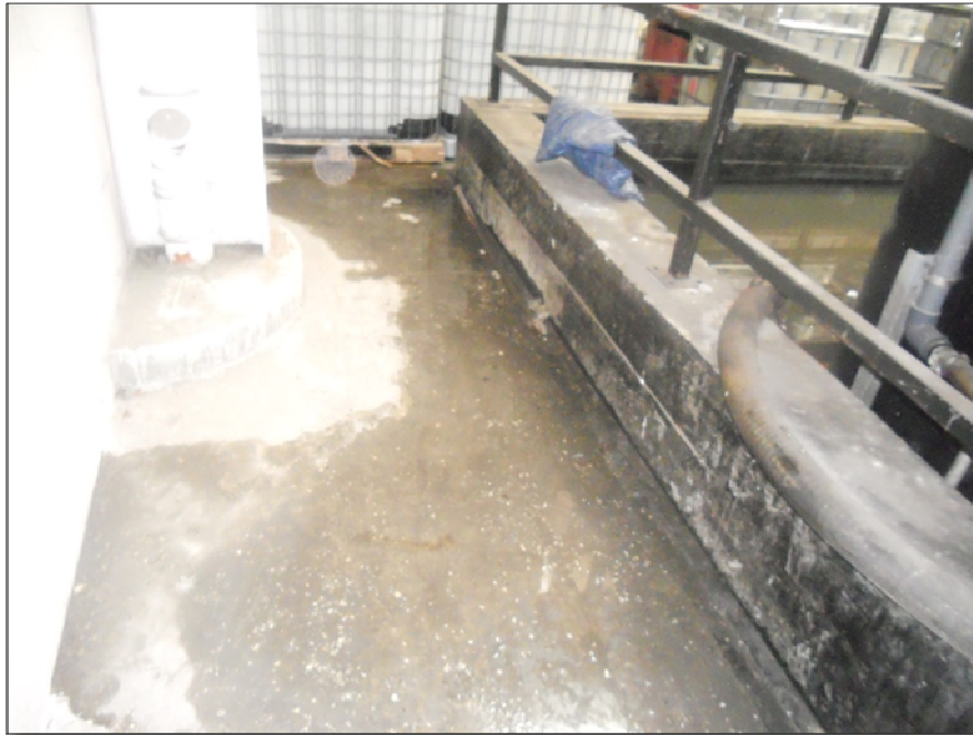
Photo 1: Suspected fault in Area / Bund No. 9
