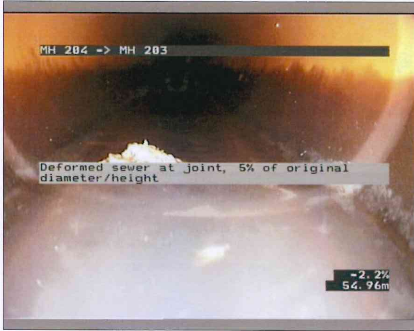
Photo: 1_5A, MPEG #: 311013_1, 00:14:48 54.96m, Deformed sewer, 5% of original diameter/height
