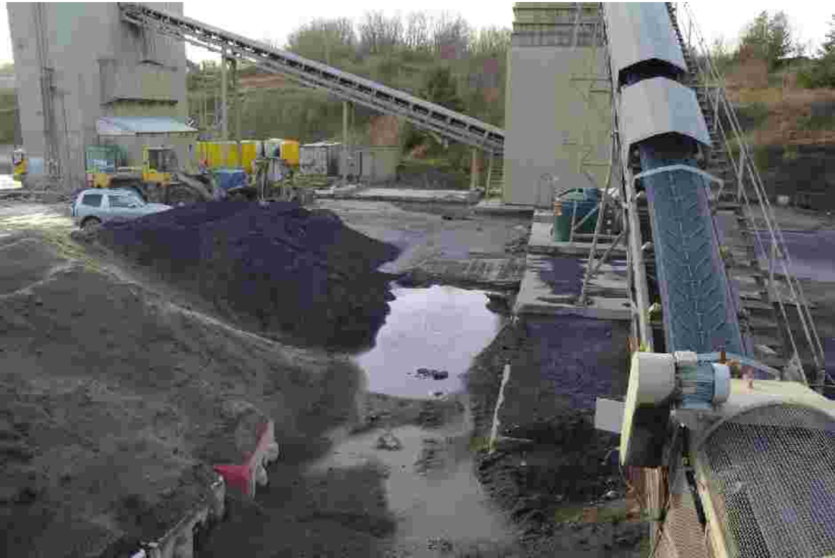
Photo 5 – Yard Drainage Impeded by Concrete Platform
