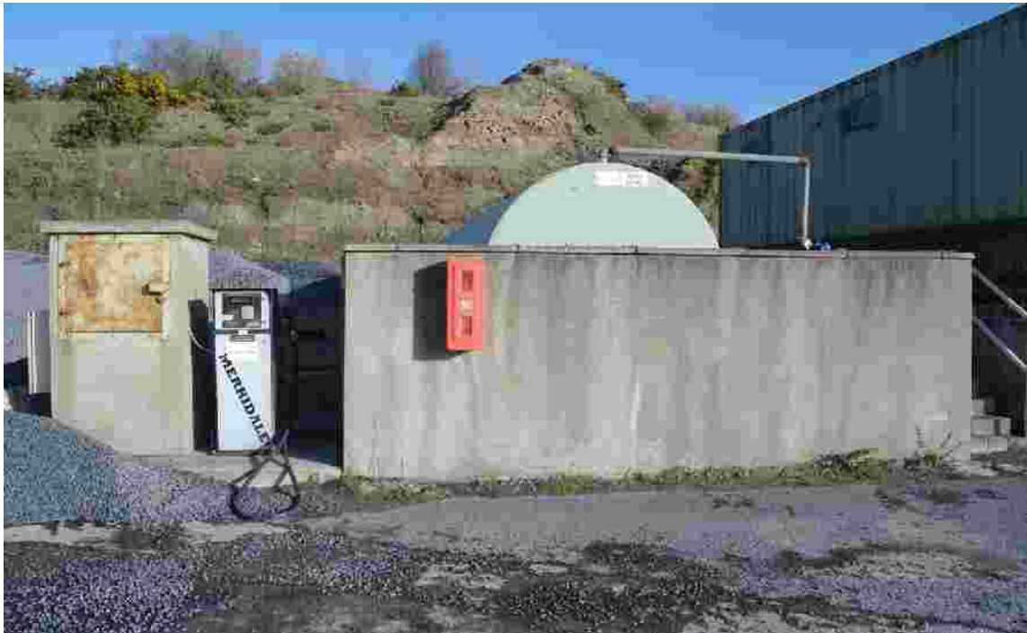
Photo 1 - Bunded 70,000 litre Diesel Tank
