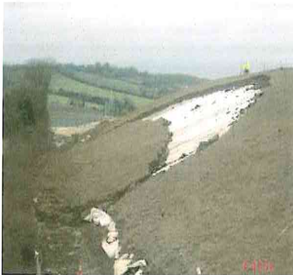
Plate 8 North West Slope Failure 2006
